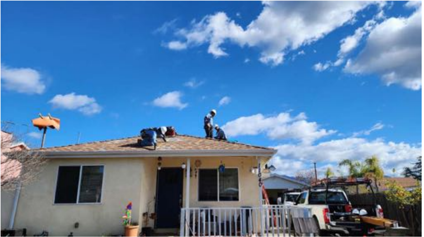
GRID Alternatives installing solar panels on a Pacoima single-family home. Photo credit: GRID Alternatives Greater Los Angeles
