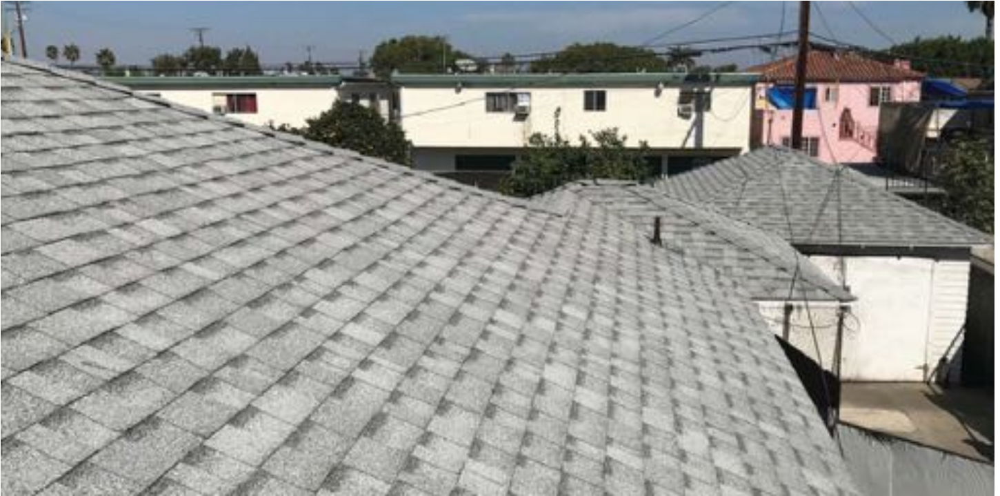
Single-family cool roof prototype offered to Green Together project area residents at no cost. Photo credit: GRID Alternatives
