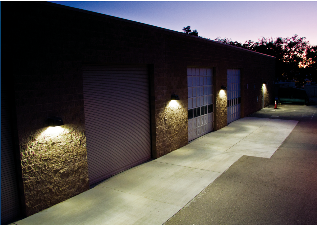
Post-retrofit network-controlled LED wall packs line the Thermal Energy Storage building at UC Davis
