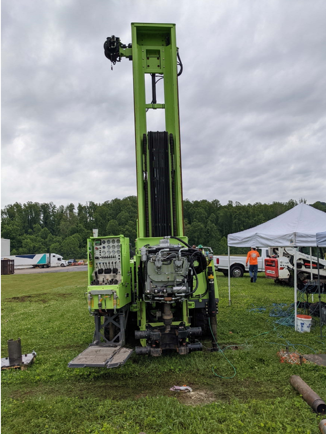
Figure 17 – Phase II rig lining up over the first boring. The SonicWands are to the right and the DAS is under the white tent.
