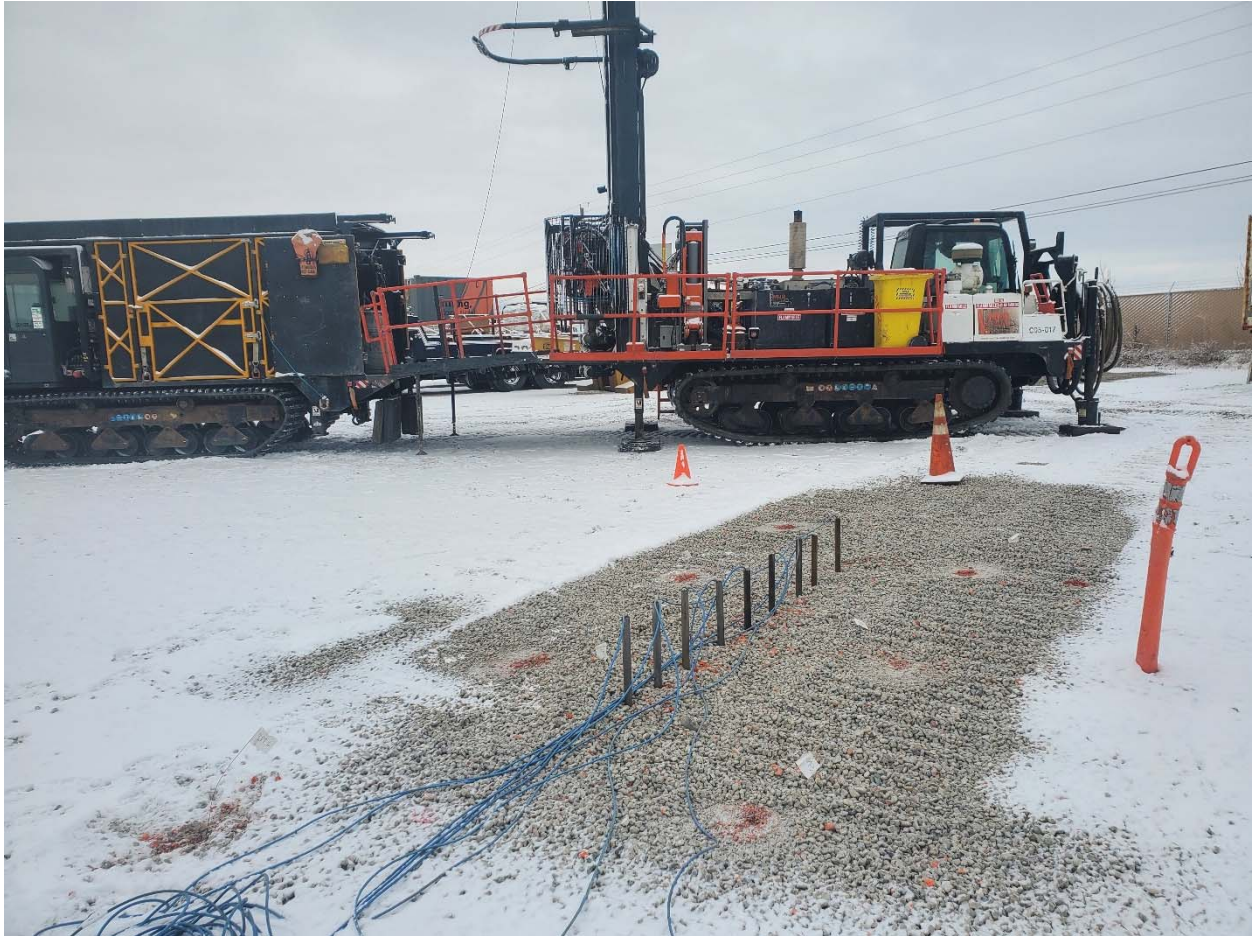
Figure 12 – Phase I field setup. The cone rods attached to the SonicWands are protruding from the subsurface. The orange markings on the ground indicate where the baseline CPTs were pushed.
