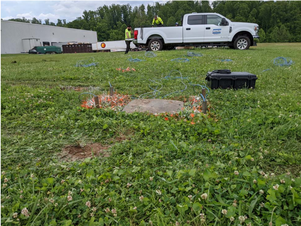
Figure 16 – Phase II stickup of cone rods attached to SonicWands. The central four SonicWands are covered by the wooden plate.
