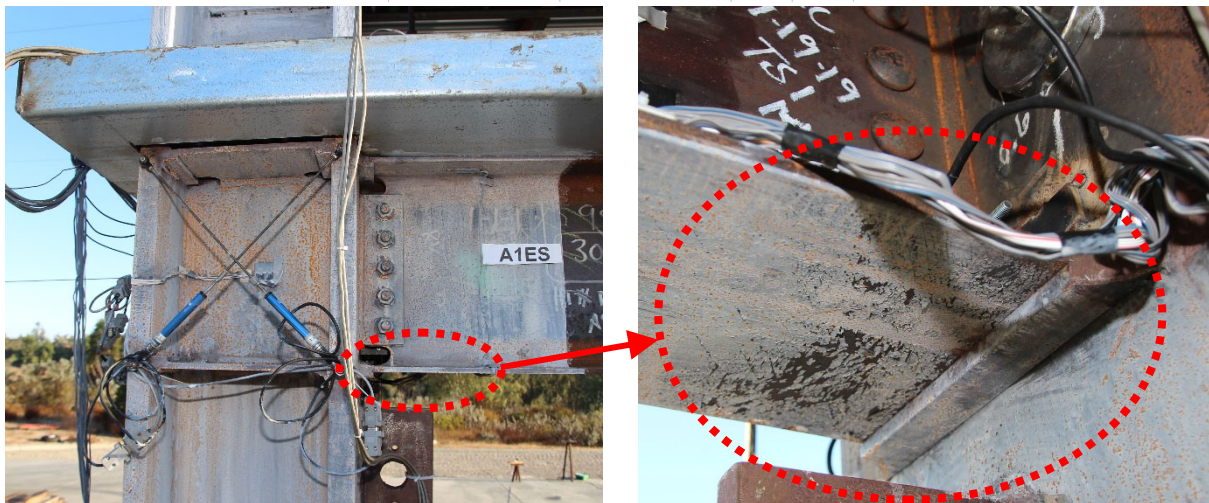
Figure 7.26 After Test 2B-3: Yielding of Bottom Flange at 2 nd Floor AFW Connections
