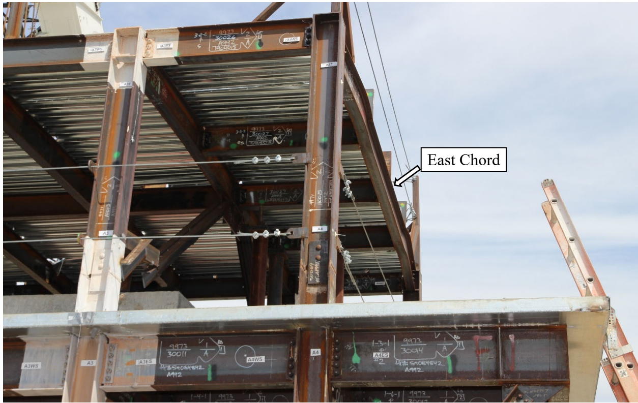
Figure 9.21 Residual Deformation of Roof East Chord
