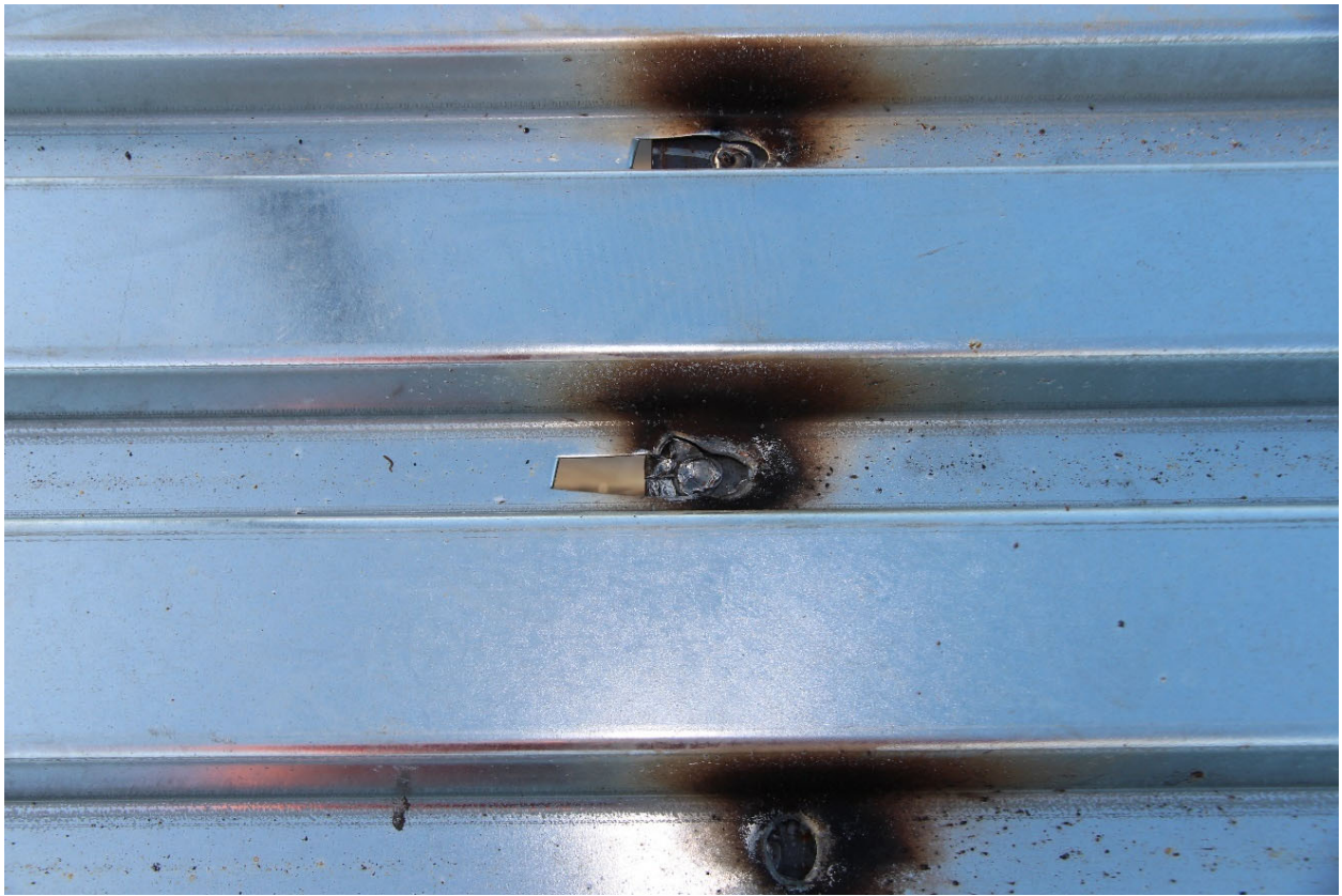
Figure 9.20 Damage of Arc Spot Welds
