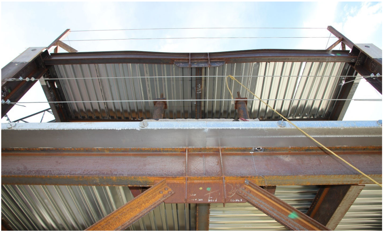
Figure 9.23 Residual Deformation of Roof West Chord
