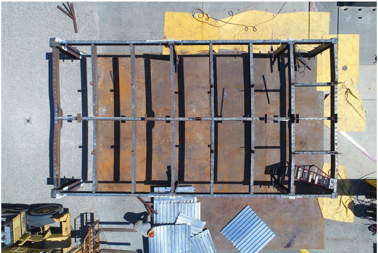
Figure 9.24 Residual Deformation of Roof Beams (after Deck Removed)
