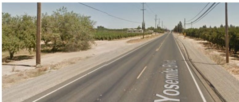
Figure A.35: On-site location photograph of PH16 (right lane) and PH17 (left lane) from Google Maps.
