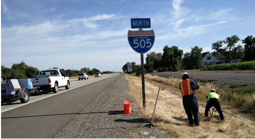
Figure A.8: PH03 on-site location photograph during falling weight deflectometer (FWD) closures.
