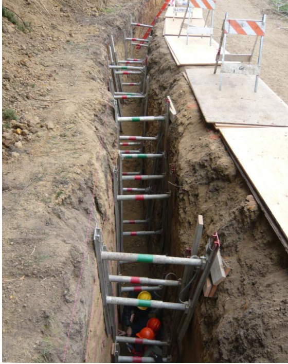
Figure 4 Geologists mapping the wall of the TR-4 trench on the Ridge Road south of LBNL excavated as deep as 4.5m and 60m long.
