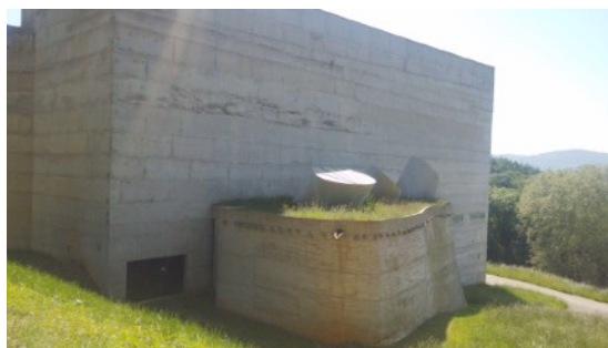
Figure 5.1 A view from north-east of the three “light cannons” protruding from the roof of the piano-shaped lower chapel at La Tourette. The wall of the chapel is an undulating concrete surface that inclines inwards toward the interior space. The church blocks most direct light from the south. (Photo by author in May 2016).
