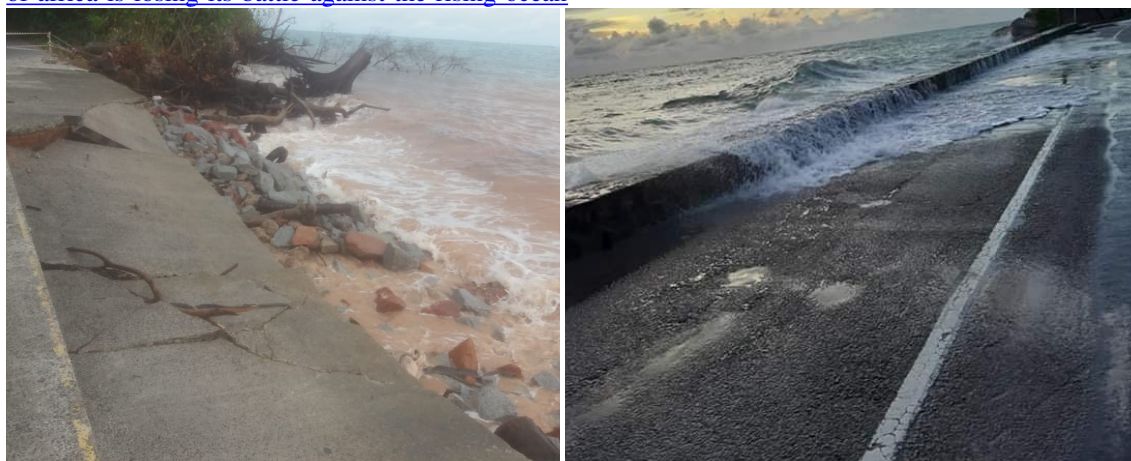
Figure 8. Saint-Louis, the old colonial capital of Senegal, faces a flooding threat that has already seen entire villages lost to the Atlantic . Source: The Guardian - https://www.theguardian.com/environment/2020/jan/28/how-the-venice-of-africa-is-losing-its-battle-against-the-rising-ocean
