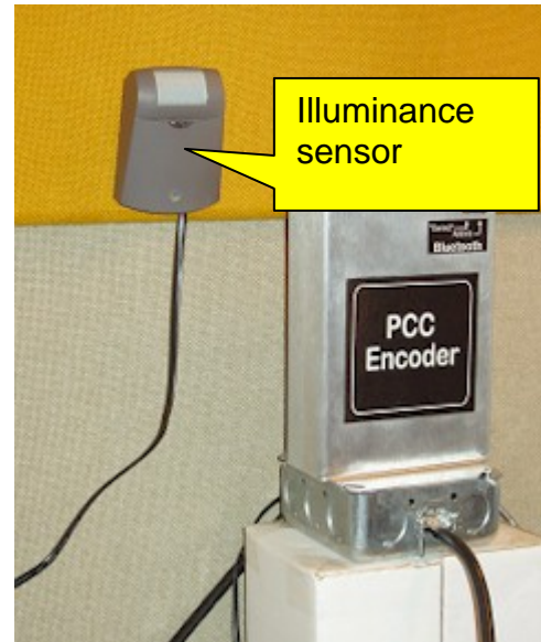
Figure 6. Closer view of the PCC Encoder and attached junction box (which collectively form the "intelligent junction box"). Also shown to the left is the environmental sensor that is attached to the wall. Note the location of the illuminance sensor within the environmental sensor.
