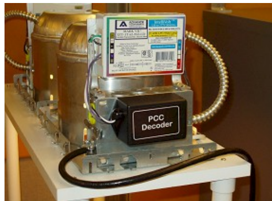
Figure 4. Closeup of the PCC Decoder and the electronic dimming ballast (0-10 VDC) controlled by the system.
