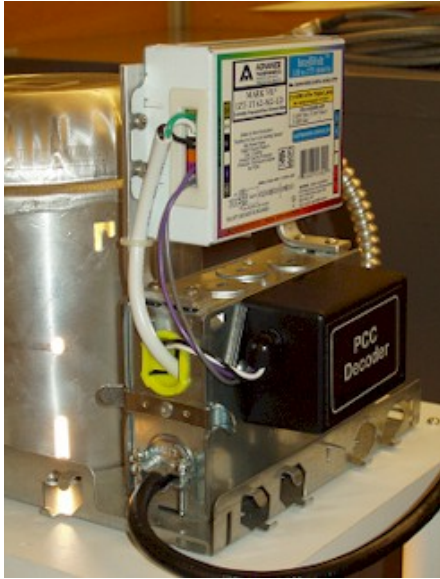
Figure 5. Closeup shot of the PCC Decoder showing the electrical connections between the decoder and the ballast.
