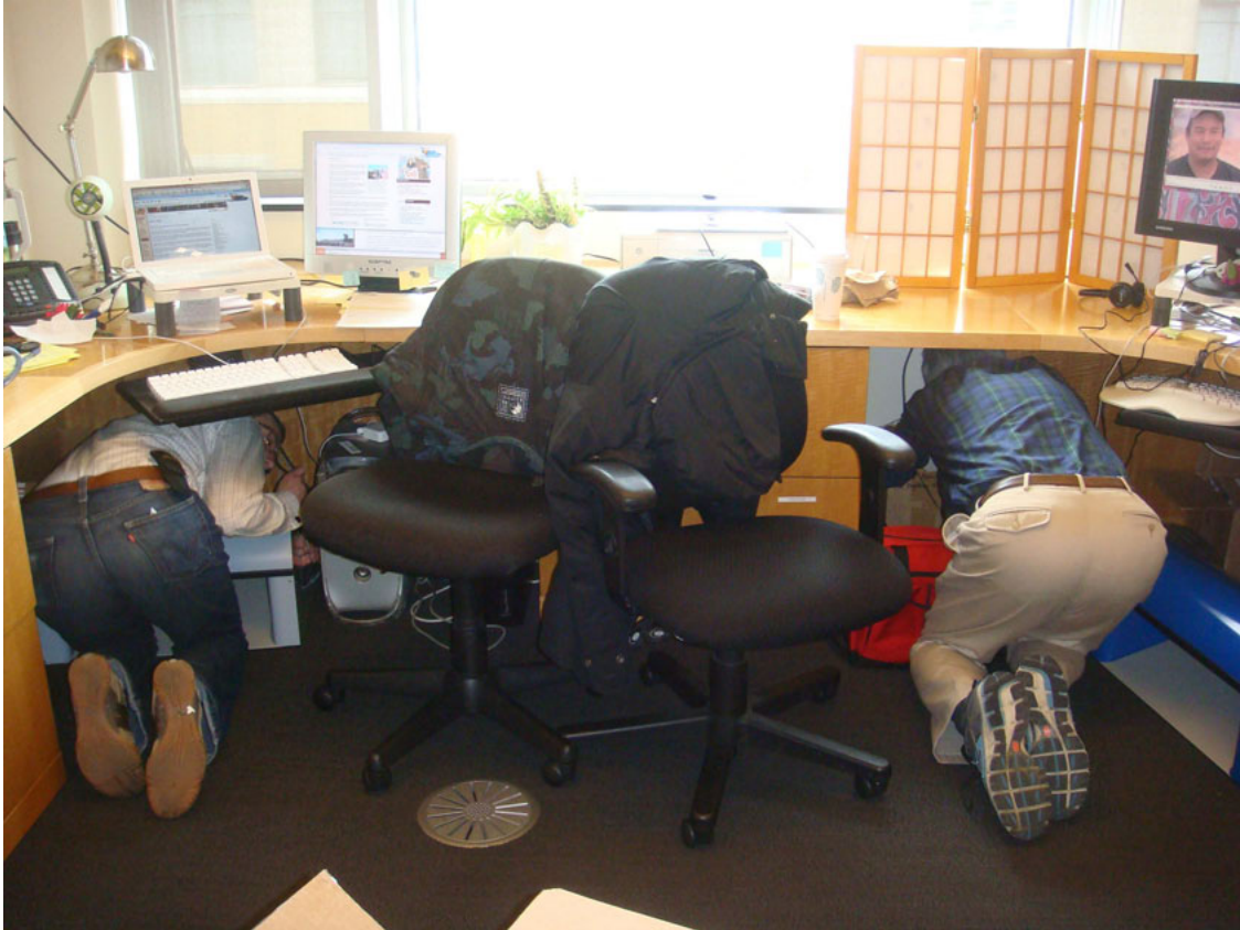
Figure 5.6: The research team installing personal control devices at a study site
