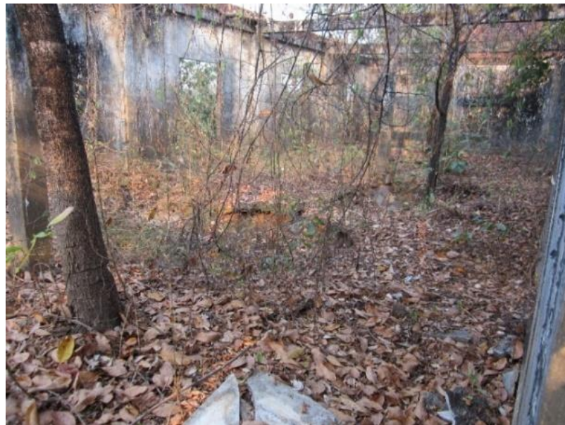
Figure 14. Interior of bombed building at Lumphat (2016). Photograph by Lina Chhun
