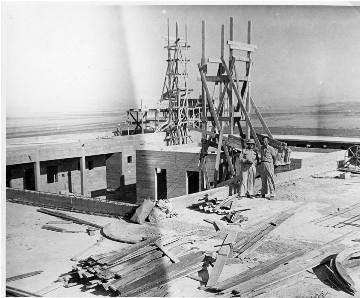
Fig. 11. The Lajjun Tegart Fort under construction in June 1940; Israel State Archive, file 58589
