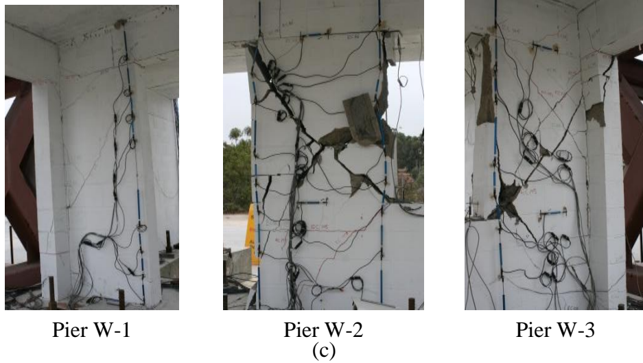
Figure 5.10 - Deformed mesh for a) negative drift, b) positive drift (the displacements are amplified by 10 times for illustration purposes); and c) actual crack pattern for the 1 st story during El Centro 160%
