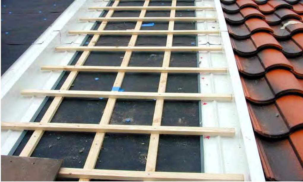
Fig. 3. Construction of the roof deck showing battens and counter-battens for attaching the slate tile and the parapets used to limit airflows on the underside of the tile to within a given test roof.
