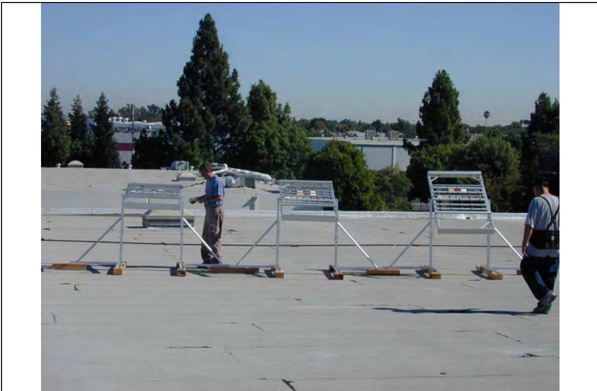
Figure A.6. Exposure rack mounted on the low-slope roof of Custom-Bilt Metal’s warehouse in Sacramento, CA.
