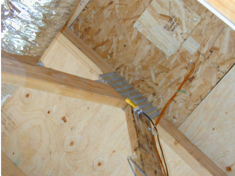
Figure 7. Instrumented sandwich panels contain thermocouples and heat flux transducer for measuring roof temperatures and heat flows.
