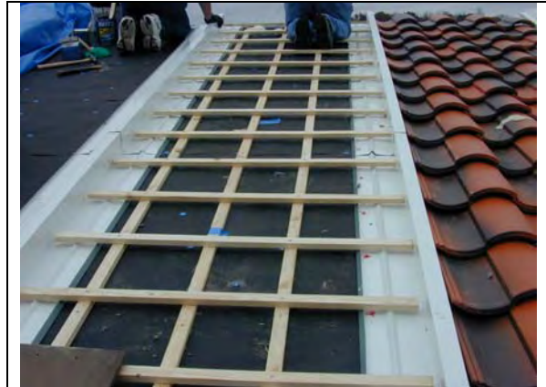
Figure 1. Batten and Counter-Batten Assembly Showing Inclined Air Cavity for the Slate Tile Roof.
