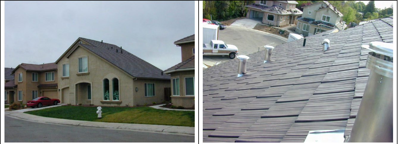
Figure 5. Finished C-style home demonstrating Custom-Bilt Metal's painted metal shake having ULTRA-Cool™ pigmented coatings by BASF.
