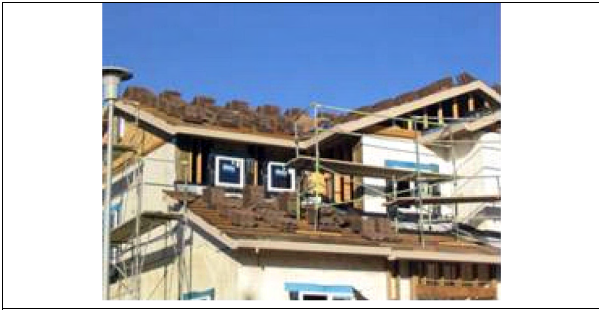
Figure 2. Hanson’s concrete tile loaded onto the roof of one of two A-style homes. The tiles were offset mounted from the roof deck using 1 in by 1 in battens.
