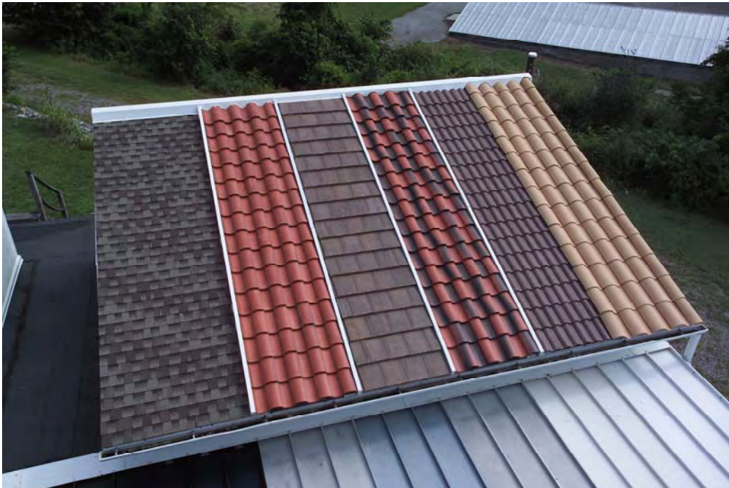
Figure 2: Clay and Concrete Tile being Field Tested on the Steep-Slope Attic Assembly at ORNL. (From right-to-left the test roofs are: direct nailed S-Mission Clay, direct nailed Medium-Profile Concrete, spot adhered foam S-Mission Concrete, batten and counter-batten Flat Concrete Slate, batten S-Mission Concrete and the direct nailed asphalt shingle roof.)
