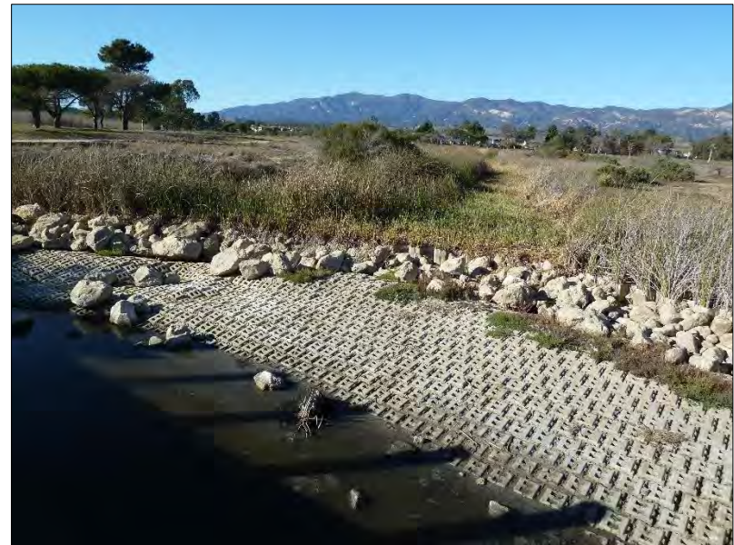
Photo 20: View north at Devereux Creek sheet pile sill separation from Devereux Slough tidal influence. 11/20/2015
