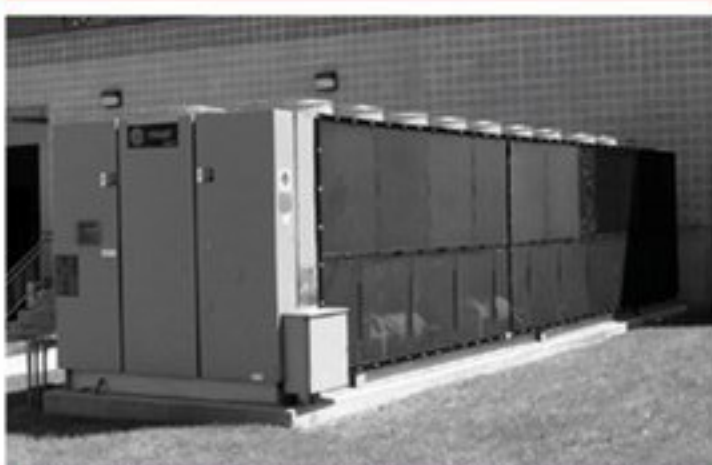
Air Cooled Chiller and Condensing Unit Filters
