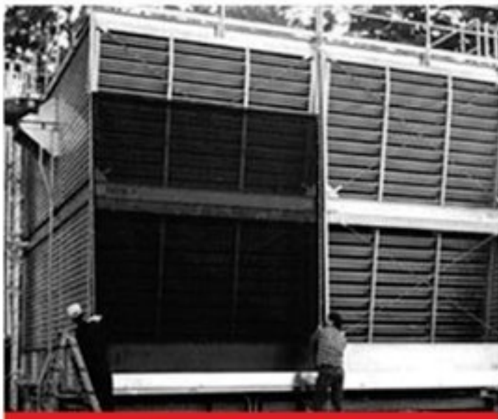
Cooling Tower Filters
