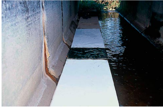
Fig. 7. Ledge for small animals in culvert with ink-method. (Photo by H. Bekker)
