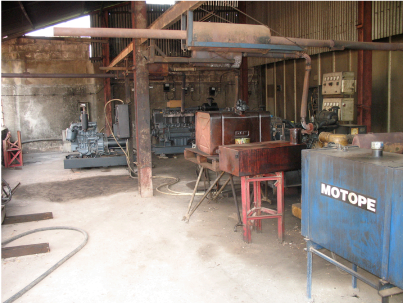
Figure 1.4: A building housing generators for an ISP in Guinea Bissau. The closest generator was poorly tuned and exhausted into the room, causing dangerous levels of carbon monoxide to accumulate in the work area.
