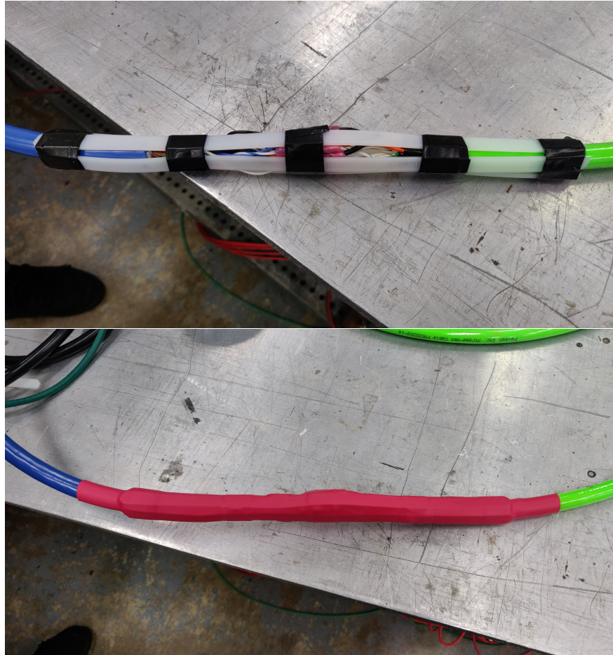
Figure A.2: TOP: Falmat cables (neon green) re-spliced with new connectors (blue). BOTTOM: Heat shrink tubing is placed over the splice to waterproof it.
