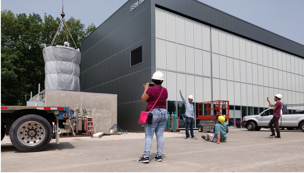
Figure 3.6: The inner structure is lowered into the experimental hall while photo shoots among collaborators take place. Plastic sheets protect the inner structure against dust during transport. The SBND (Short-Baseline Near Detector, as part of the Short-Baseline Neutrino Program) experimental hall is the large building to the right.
