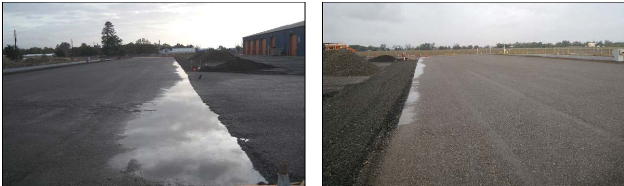
Figure 2.23: Ponding of water on base.
