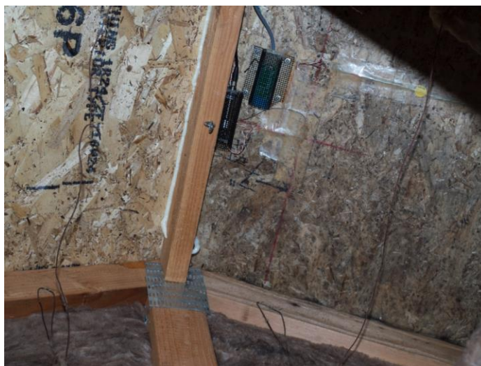
Figure 9. Clovis test home, photo of mold growth on North-sloped OSB roof deck (right side)
