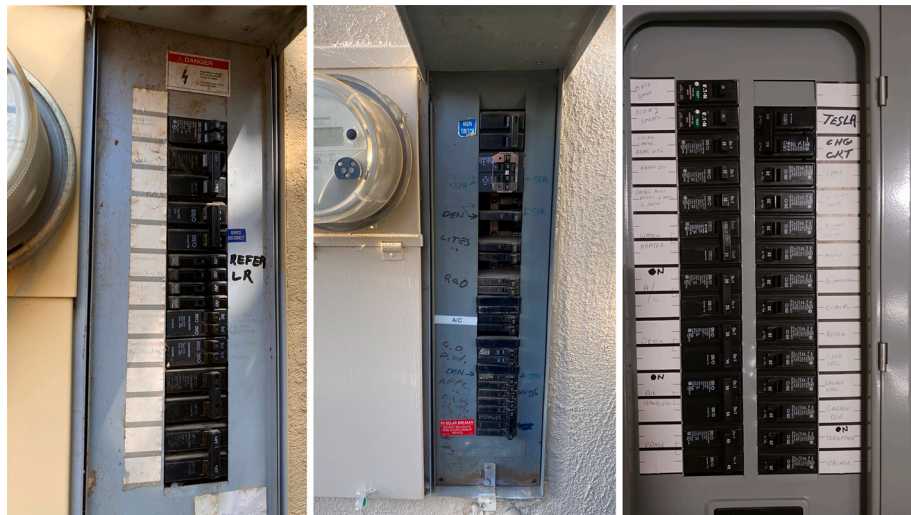
Fig. 13. Variability in Circuit Breaker Labeling. These panels show the range of labeling practices found in our survey.
