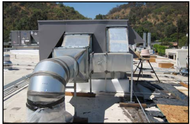
Rooftop HVAC Unit
