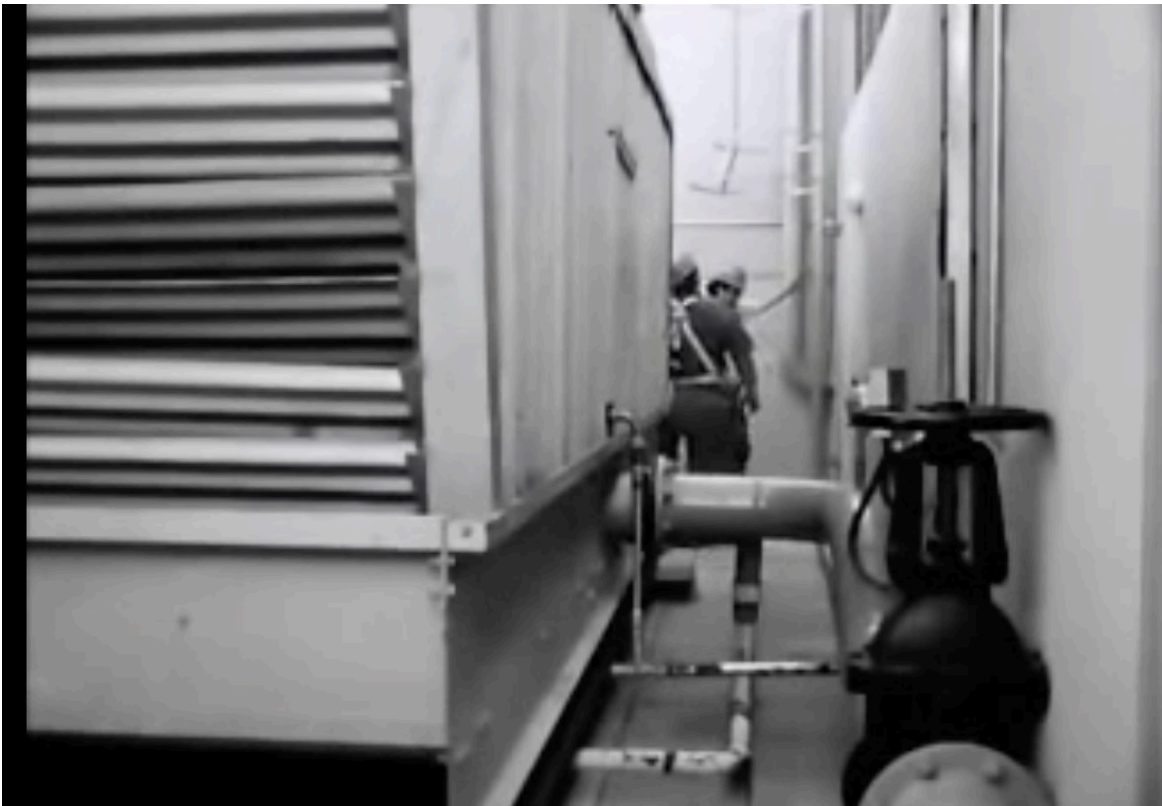
Figure 3.1: Pipe-laden infrastructure in Mundo Grúa
