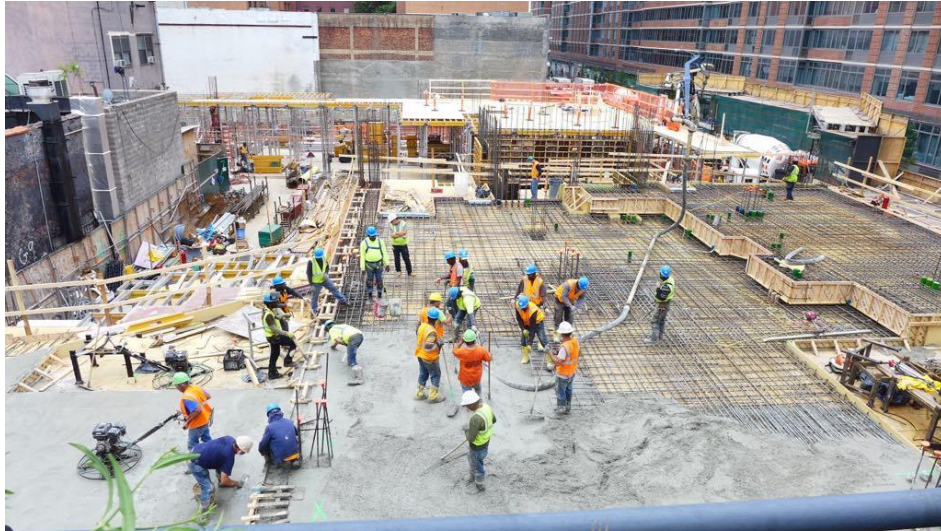
Fig. 3. Construction site for 528 West 28th street, Zaha Hadid, June 2015. View from the High Line, Chelsea. With the opening of the High Line, New York City re-zoned West Chelsea in 2015, commencing in a high-end real estate boom. This photo witnesses the birth of the fabulous condominium complex designed by the late architect at 528 West 28th Street. Photo Credit: Denice Martone.
