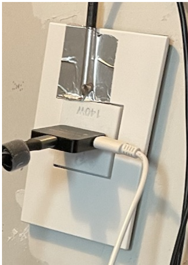
Fig. 4. The outlet mounted in a wall section with a PowerZ USB tester plugged into it.
