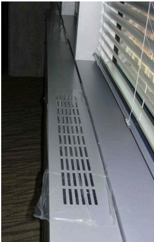
Figure 13: Sealed perimeter linear grilles
