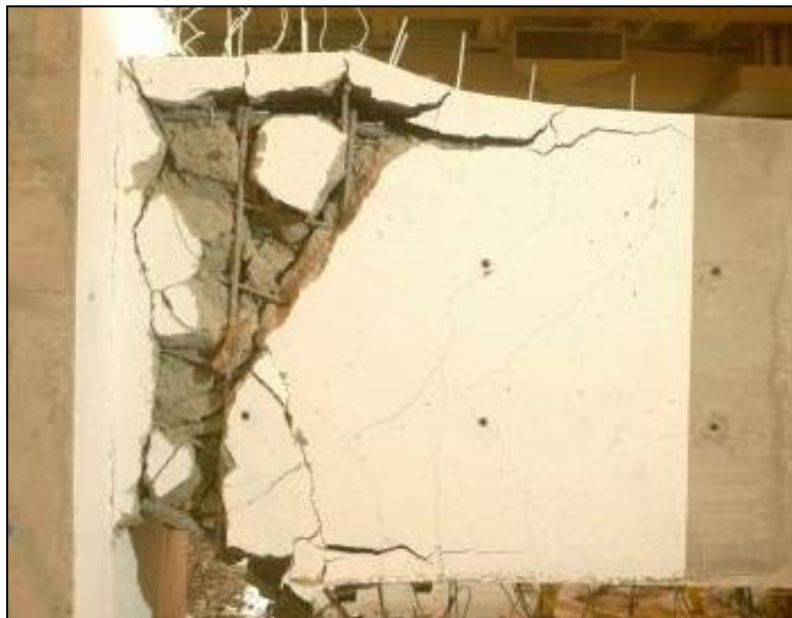
Figure 2.7.3. Buckling of bottom longitudinal bars and large apparent shear deformation in Beam 1 (cycle with peak \theta = 0.055 ).
