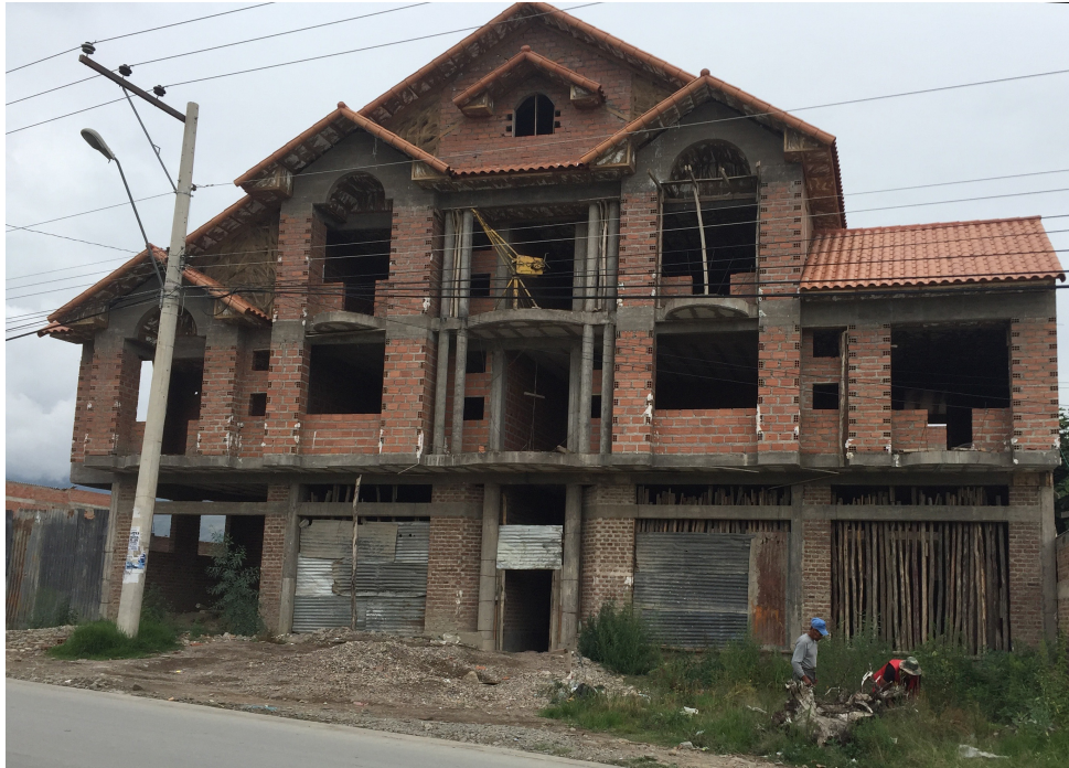
Figure 6.1: House under renovation in semi-periphery town of Quillacollo (near city of Cochabamba) (photo credit: Amy Kennemore)
