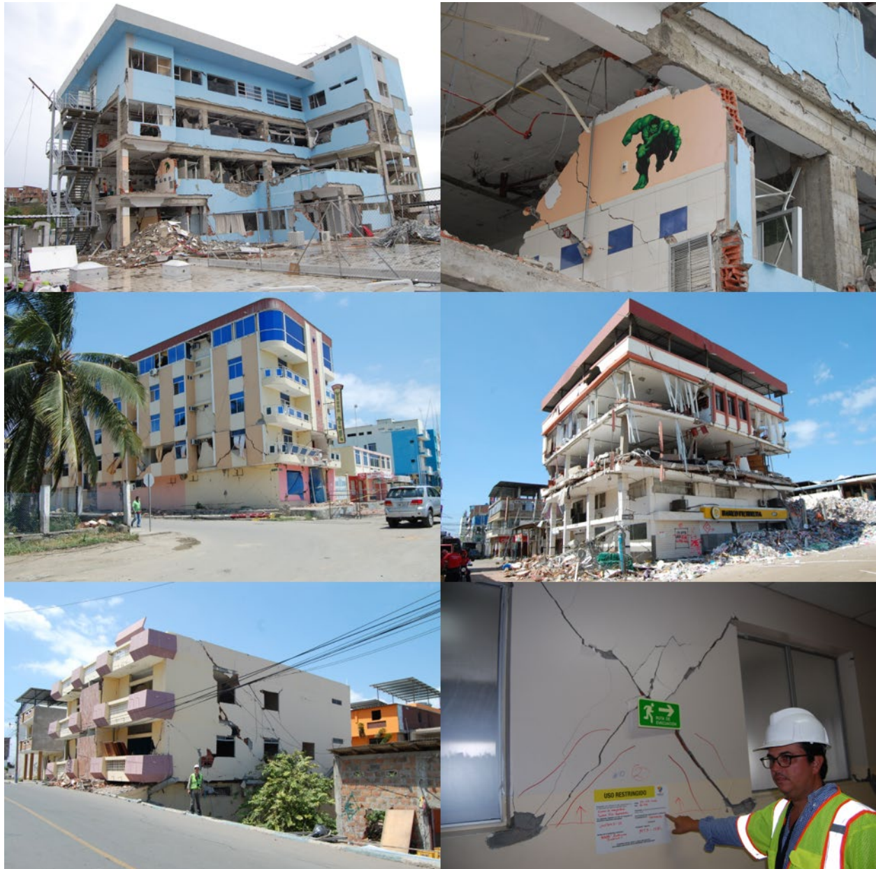
Figure 1.6 Examples of observed damages on RC frame buildings with URM infill walls after the 2016 Muisne earthquake (photos by C. Arteta).
