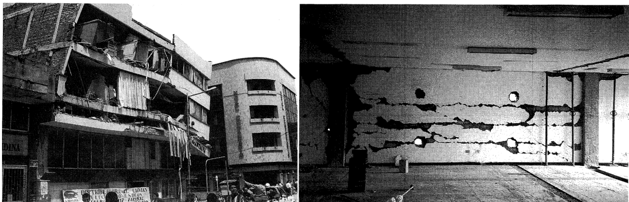
Figure 1.3 Examples of poor performance of RC frames with URM infill walls buildings. Adapted from Restrepo and Cowan (2000).
