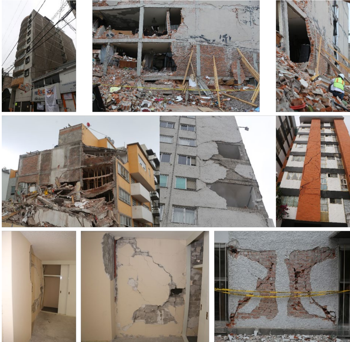
Figure 1.9 Examples of observed damages on Unreinforced Masonry infill walls (photos by J. Archbold).
