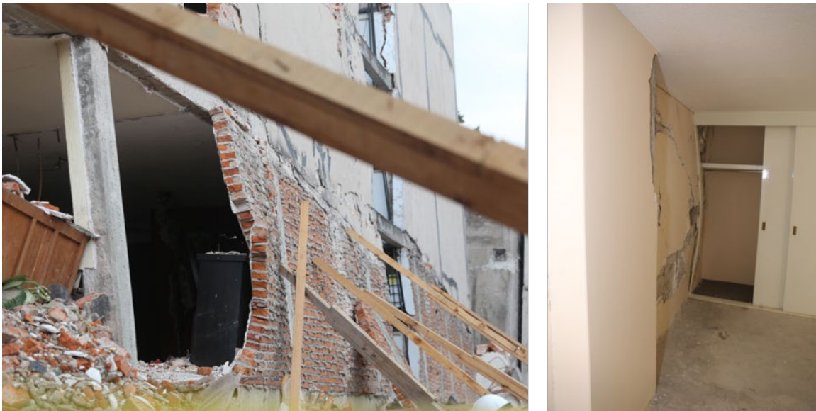
Figure 2.8 Examples of observed out-of-plane damage of URM infill walls after the 2017 Puebla earthquake (photos by J. Archbold).
