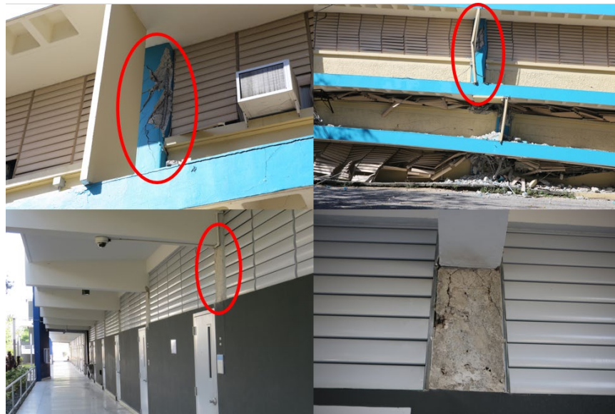
Figure 2.3 Buildings with concentrated shear damage in columns due to captive column effect following the 2019-2020 Puerto Rico earthquake sequence. (photos by J. Archbold and A. Messina).
