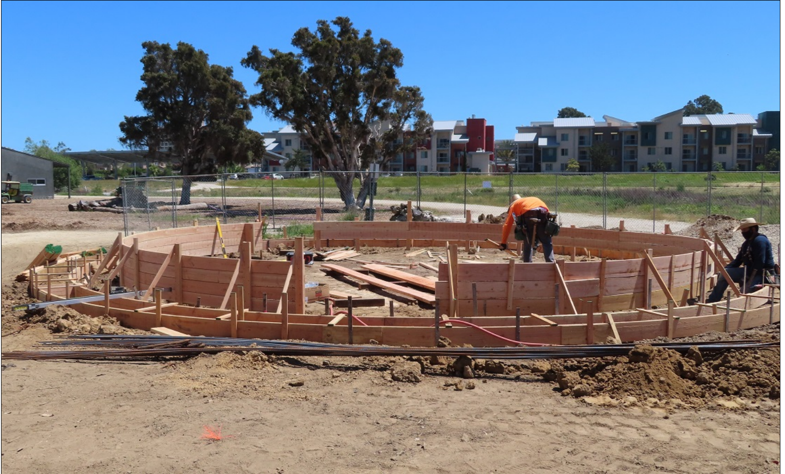
Contractors installing a temporary frame for constructing the foundation of the NCOS visitor plaza.
