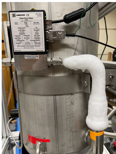
Figure 6a shows the ice forming on the nitrogen recirculation line, where ice starts from the end of the vacuum jacket and stops before the flow meter.
