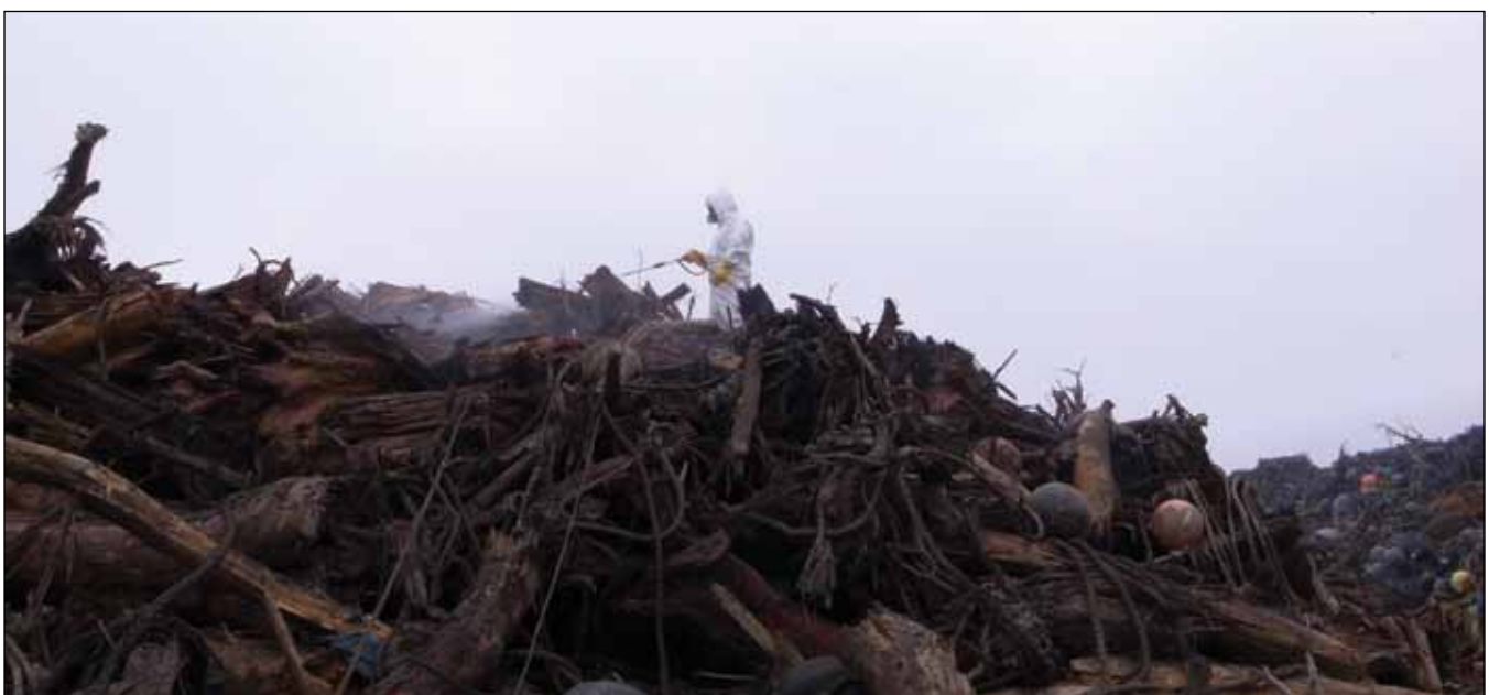
Plate 12: A high-risk job – a technician applying insecticide at the top of a hill-high rubble heap.
