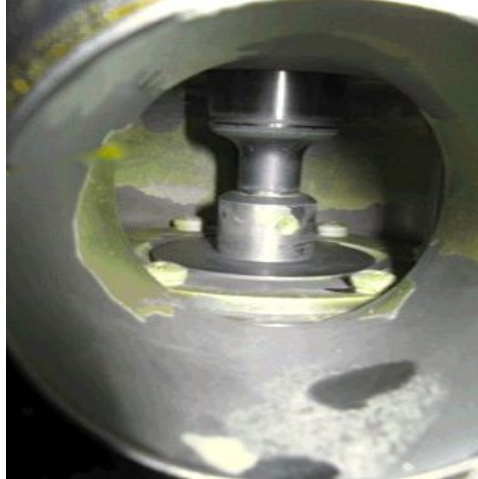
Figure 3.3: Image of sulphur contamination (yellow deposits) of fuel control valve. (Courtesy Solar Turbines Inc.)
