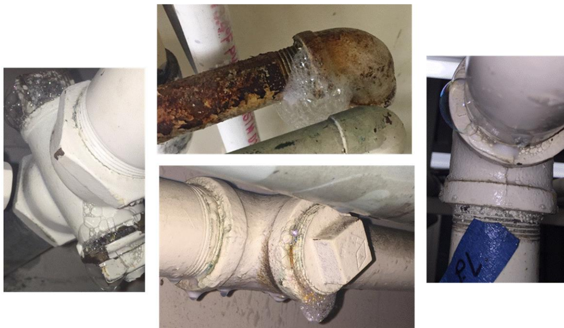
Figure 14: Images of various detected NG leaks within the test infrastructure
