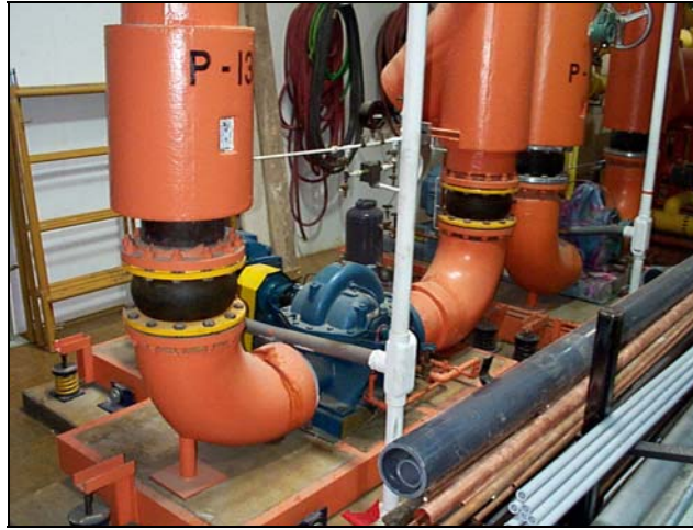
Figure 4. Hot Water Pumps
