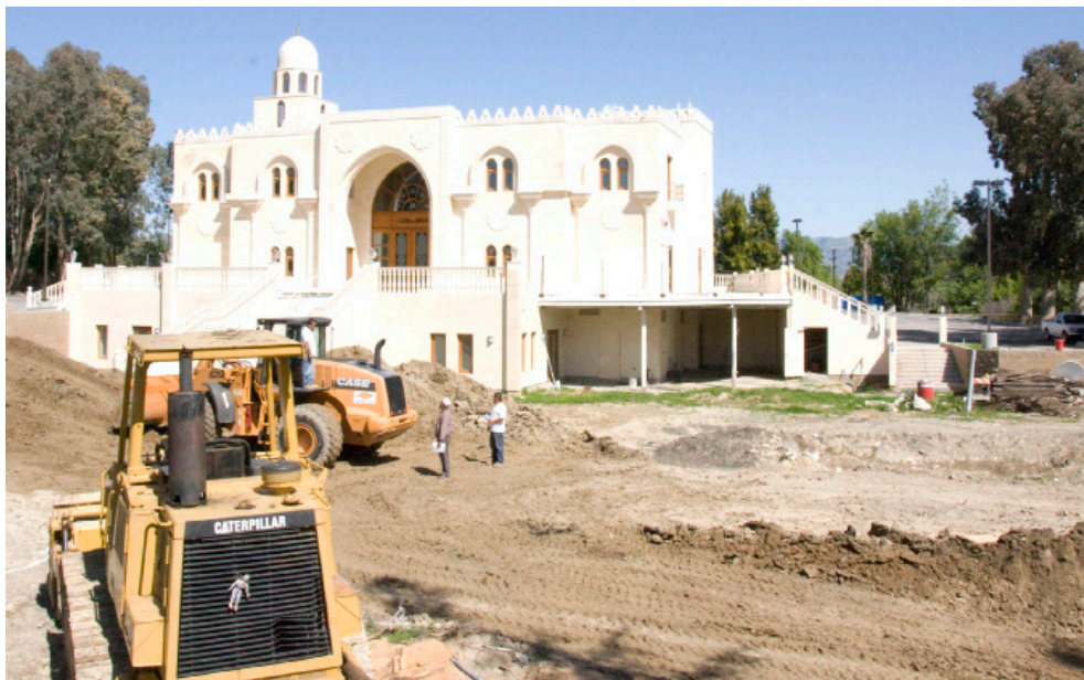
Figure 33: Excavating below the surface-level to conform with the City's municipal code. Source: Courtesy of Najam Alanwar.
