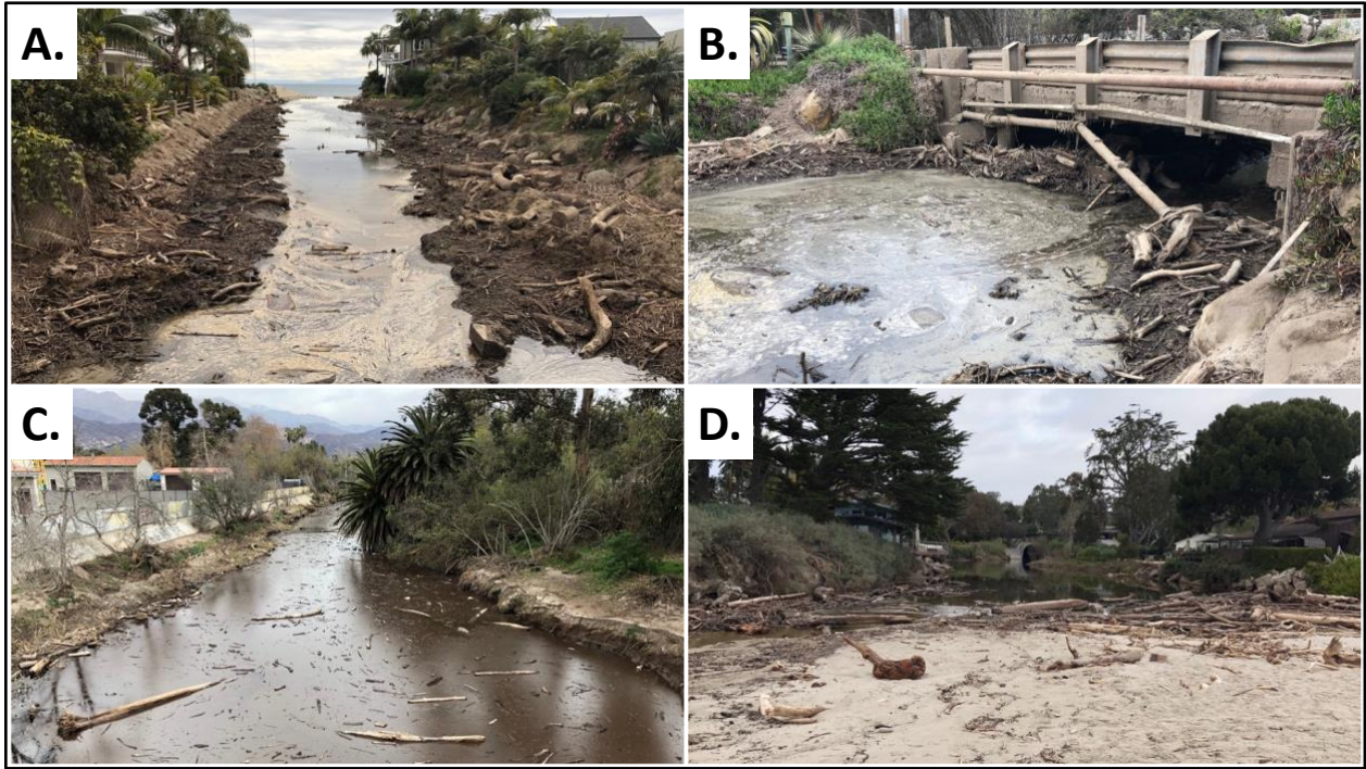
Figure 3-7. (A-B) Arroyo Paredon, Santa Barbara County. (C) Carpinteria Creek, Santa Barbara County. (D) Rincon Creek, Ventura County. Photos taken on March 1, 2018 post Thomas fire debris flow. Note that the Thomas fire affected multiple systems simultaneously. Additional modeling effort will be required to account for the apparent increased frequency of large fire events and other episodic regional impacts that simultaneously affect multiple systems. Such dynamics are not considered within the current model framework.
