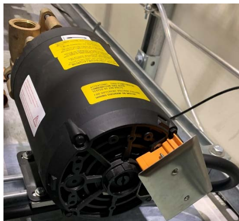
Figure 6.21 – Cold Water Pump.
