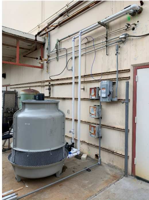
Figure 6.22 – Exterior Cooling Water Loop with Cooling Tower.
