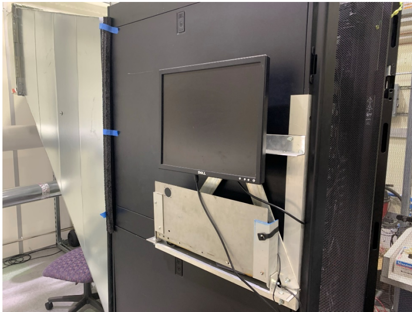
Figure 6.37 – Server Rack Computer Workstation.
