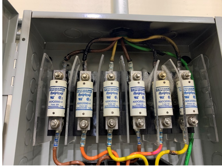
Figure 6.32 – Electrical Failure in Heater Fuse Enclosure.
