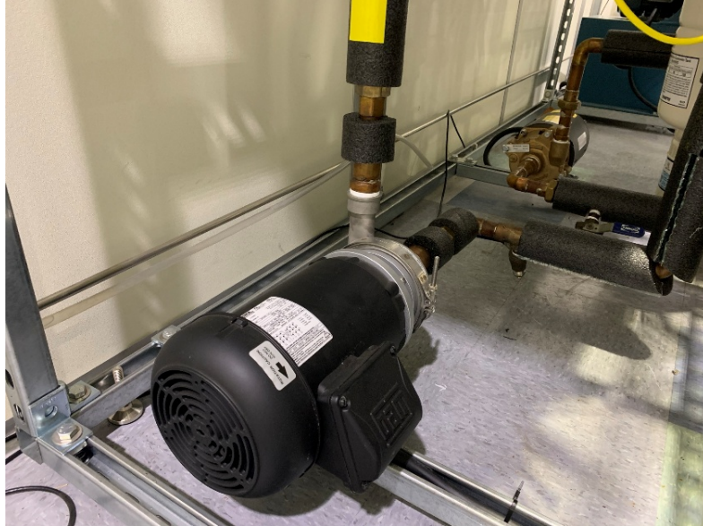
Figure 6.18 – Hot Water Loop Pump.
