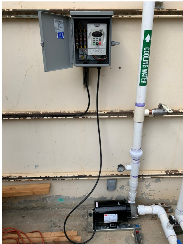
Figure 6.25 – New Cooling Water Pump with VFD.
