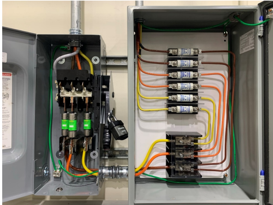
Figure 6.33 – Renovated Fuse Enclosure Layout.
