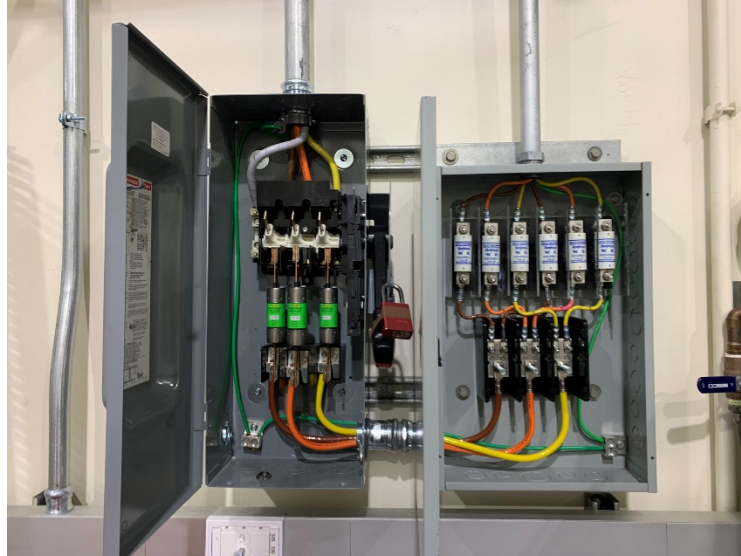
Figure 6.31 – 480 V Disconnect, Distribution Block, and Fuse Blocks.
