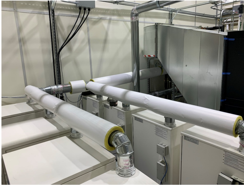
Figure 6.11 – Modified BlueGEN Exhaust Manifold.
