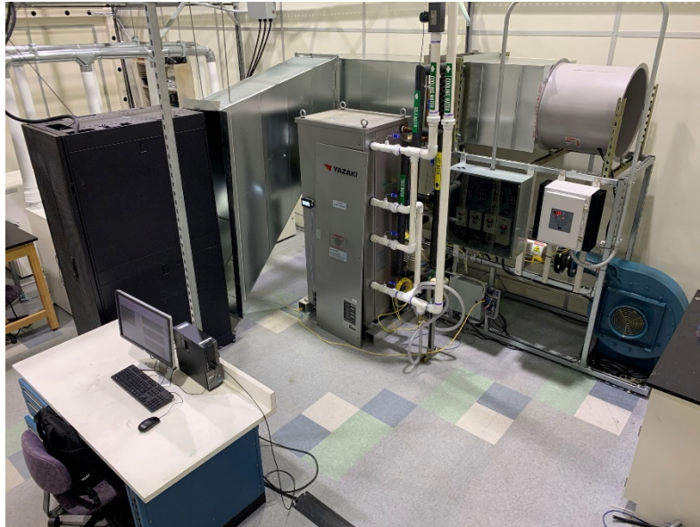
Figure 6.39 – Process Air Ducting Installed on Absorption Chiller Test Stand.
