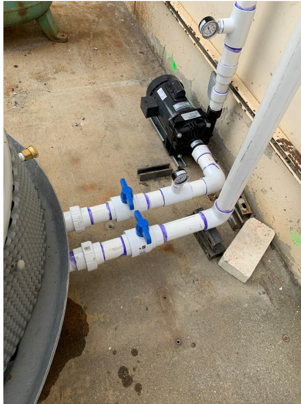
Figure 6.24 – First Cooling Tower Pump.
