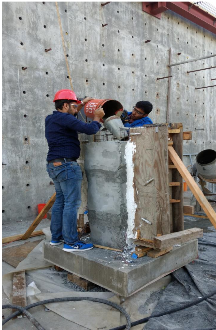
Figure (3.11): Mortar Poured from the Top to the Inner Faces of Column-Wall Connection
