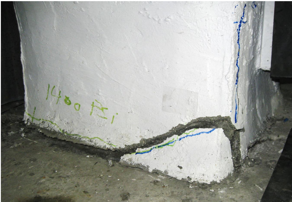
Figure (3.31): Large Cracks Observed at the Column-Footing Joint of I-section Column
