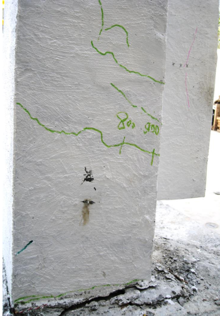
Figure (3.35): Cracks Observed on the Mortar Surface of C-section Column
