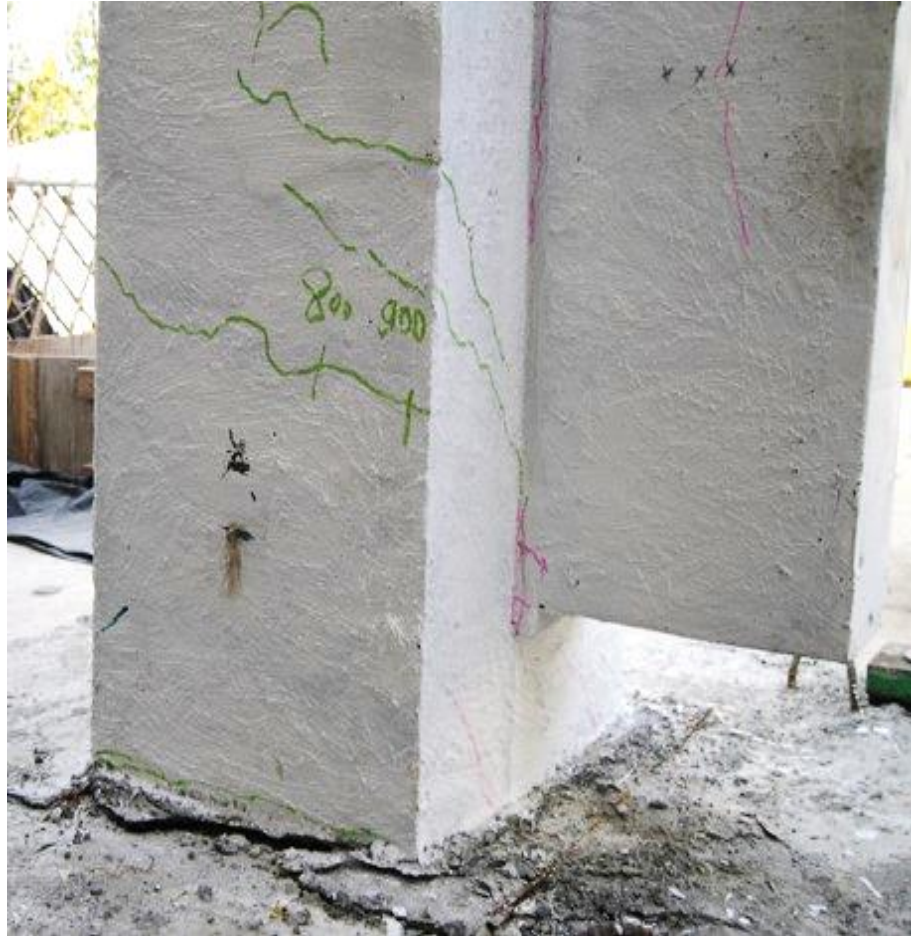
Figure (3.30): Crack Patterns for Composite C-Section Column
