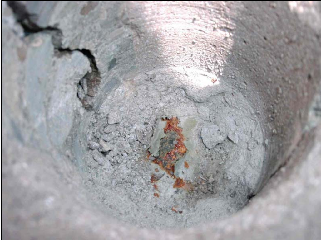
Figure 55. View of the interior of a recently made core hole showing corrosion products underneath the epoxy coating.
