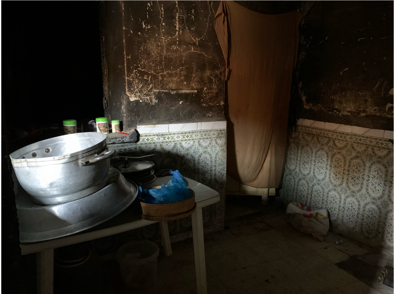
Figure 1.8 Inside the burned portion of the house. Photographed by author, August 2019.
