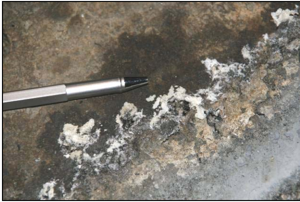
Figure 4.14: 604FD: Crystallized salt on edges of wheelpaths during testing.
