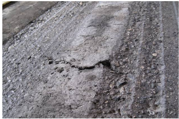
Figure 4.29: 605FD: Cracks in wheelpaths during testing.
