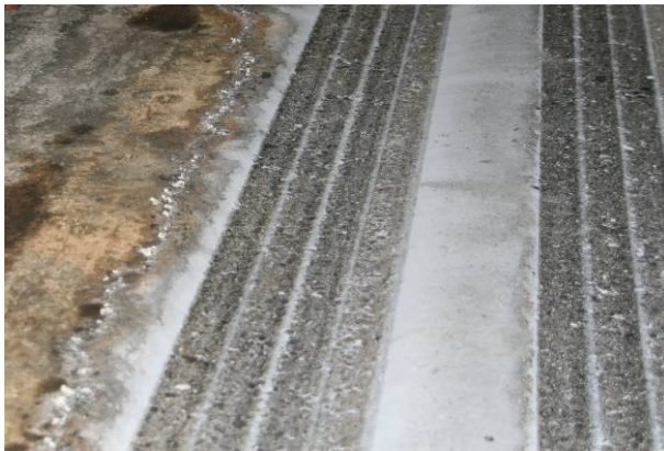
Figure 4.28: 605FD: Crystallized salt on edges of wheelpaths during early testing.
