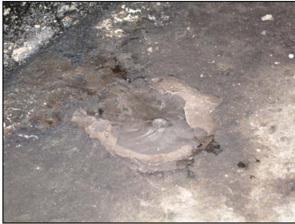
Figure 4.31: 605FD: Fines pumped from holes drilled for presoaking.
