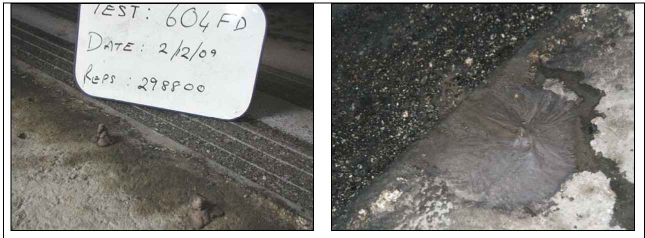
Figure 4.17: 604FD: Fines pumped from holes drilled for presoaking.
