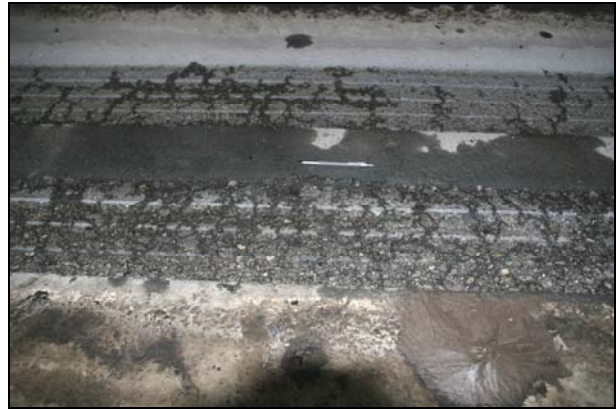
Figure 4.15: 604FD: Cracks in wheelpaths during testing.
