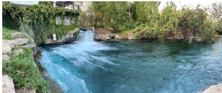
Figure 29: The spillway at Headwaters swimming area below the Burluson Dam. Looking upstream. Photo taken by Lilly Byrd, Nov. 14, 2020.
