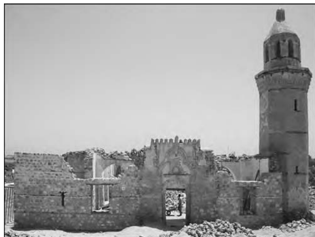
Figure 26.3. The Shafai Mosque in Suakin during restoration work in the spring of 2010. Built in the 17th century CE this mosque is the largest on Suakin Island. It was in a serious state of disrepair and its restoration, implemented by the National Corporation of Antiquities and Museums with funding of the British Embassy in Khartoum, is an important step towards the future recognition and rescue of Suakin's cultural heritage.
