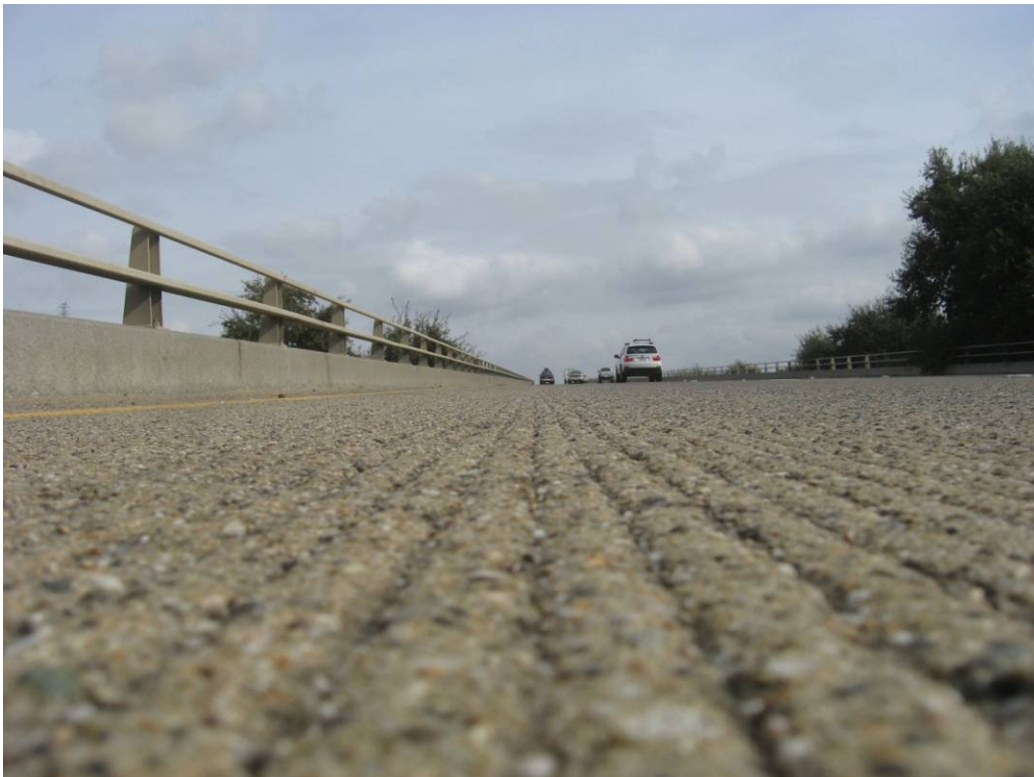
Figure 4.121: Detail of longitudinal texture on polyester overlay deck on Section QP-151.1.
