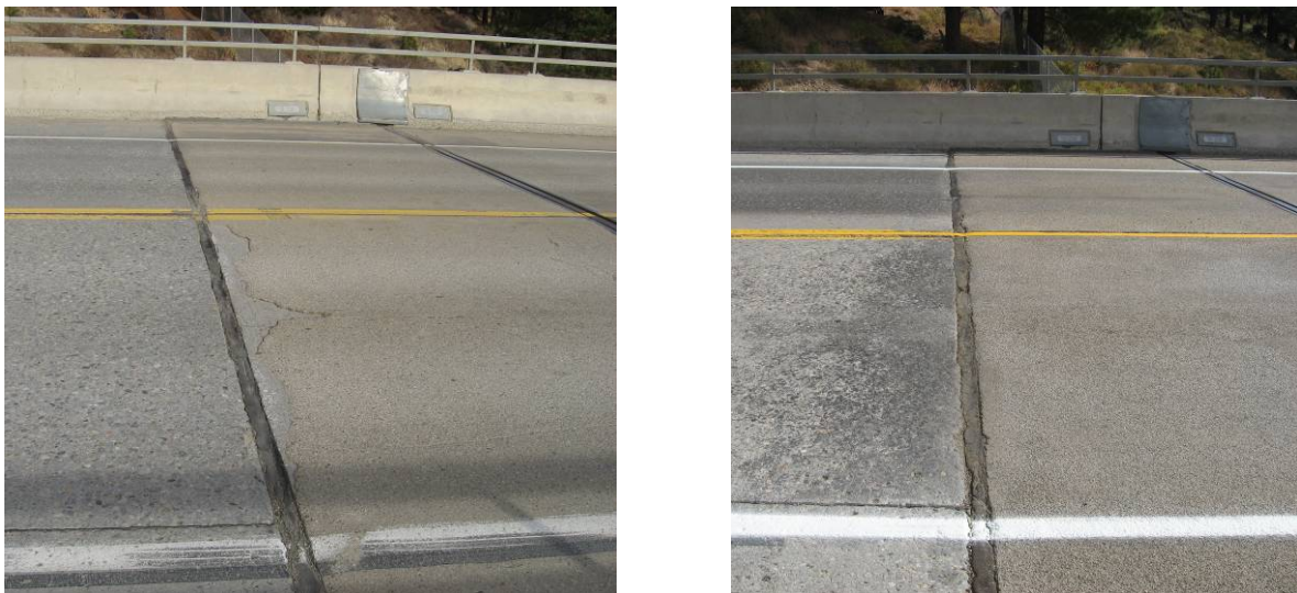
Figure 4.98: Beginning of Section QP-145.1 (right side of photos), Year 1 (left) and Year 2 (right).
