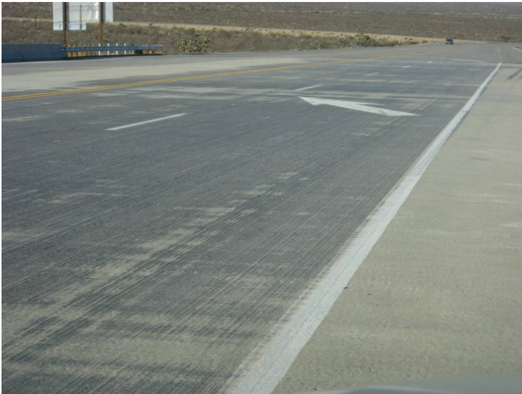
Figure 4.159: Overall view of texture on Section QP-165.1.
