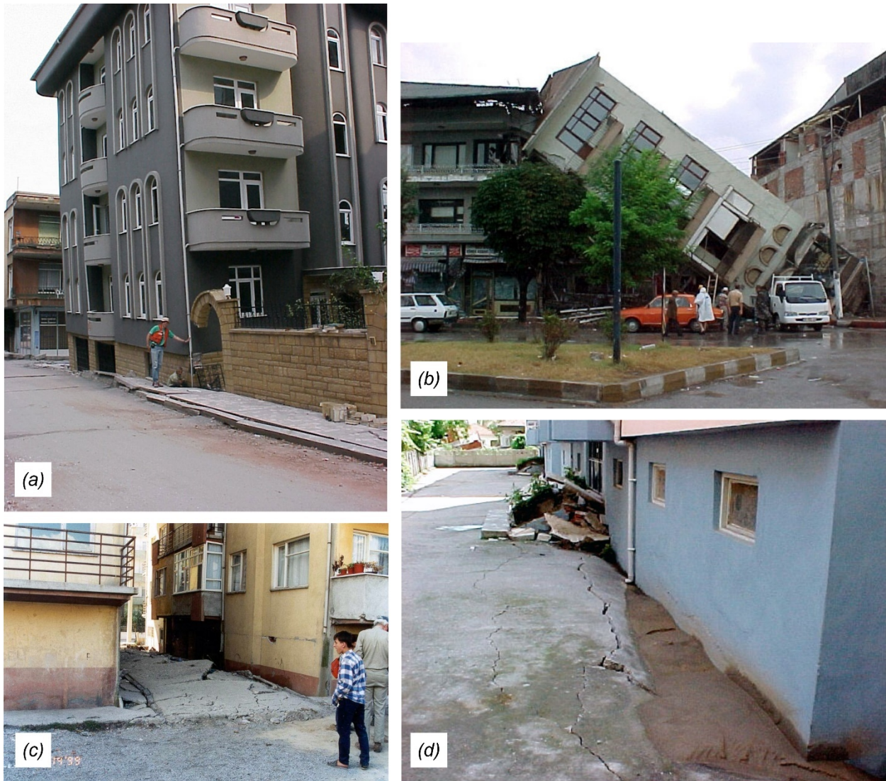
Figure 6.2. Examples of structural and ground failure in Adapazari – Turkey during the Kocaeli 1999 earthquake (photos from PEER: http://peer.berkeley.edu/publications/turkey/adapazari/ ); (a) 1.5 m of settlement of a 5-story building, (b) overturning of a 5-story building, (c) ground distress in between two buildings, and (d) structural settlement and sand ejecta next to a building
