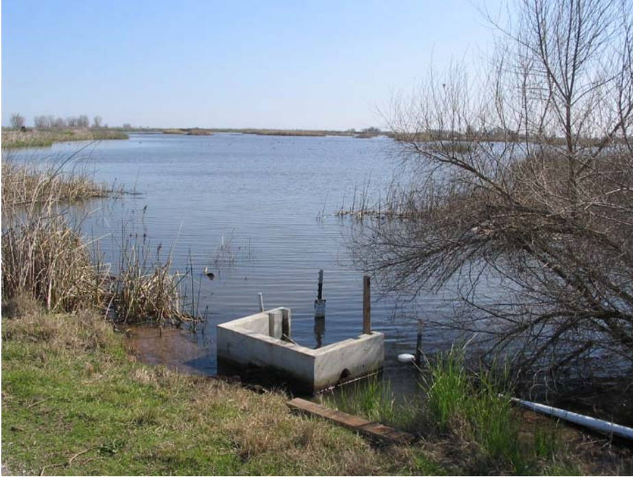
Figure 3-10: Los Banos Wildlife Management Area pond 33 outlet weir.
