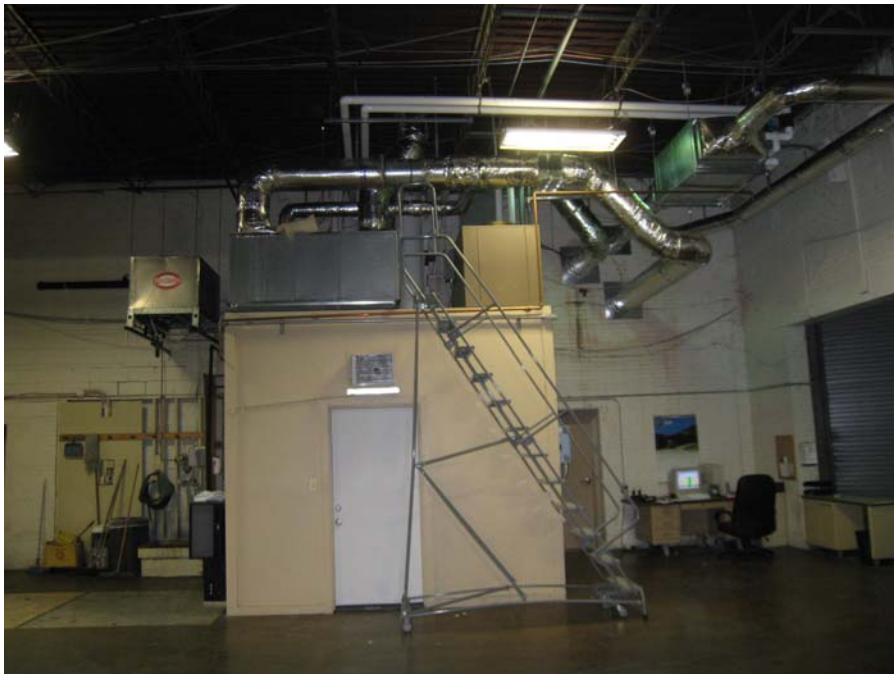
Figure A3: HVAC equipment for the test chamber and EC
