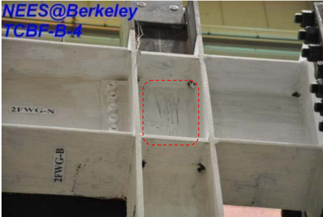
Figure 4.418 Panel zone yielding in the roof beam to column connection region
