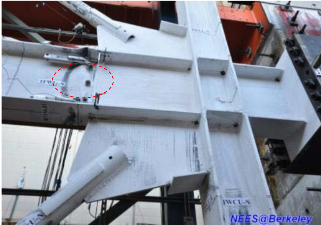
Figure 4.211 Local buckling of lower beam web at west side (Specimen TCBF-B-2)
