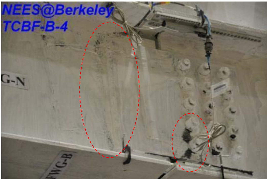
Figure 4.417 Additional flaking of whitewash near the lower beam splice plate
