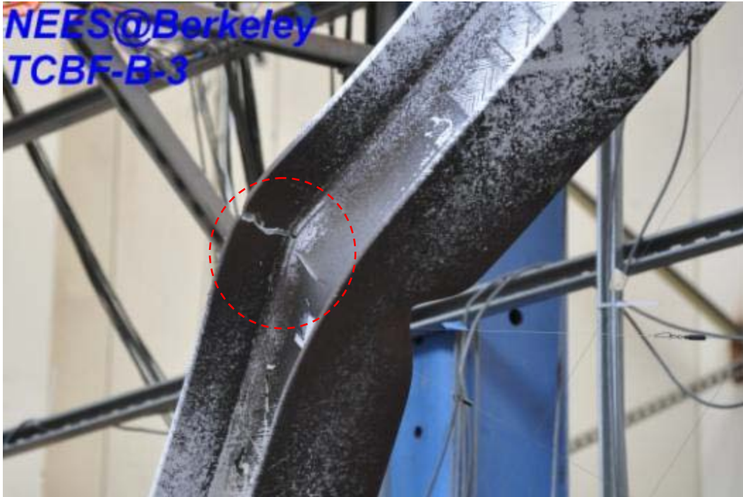
Figure 4.325 Top flange of the west wide flange brace completely fractured near the middle of the brace (view from north-west side)
