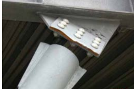
(b) Detail view of a brace connection fracture in a two-story parking structure
