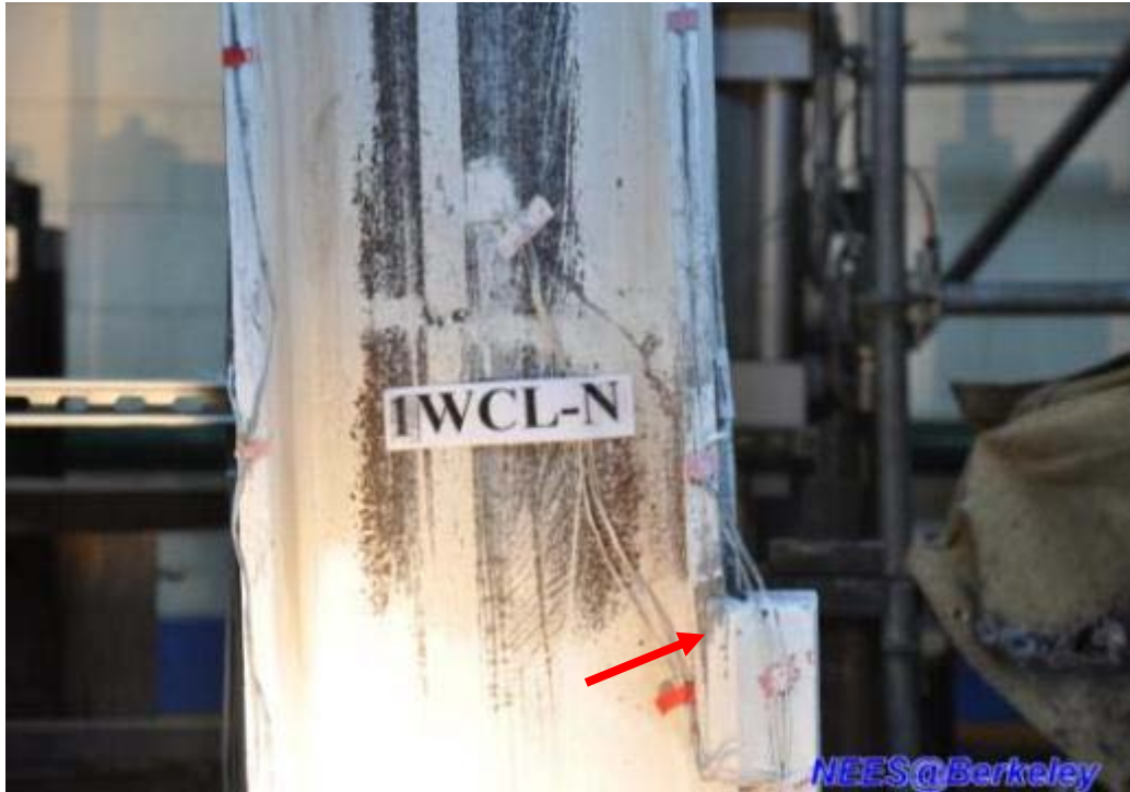
Figure 4.213 Tearing of the vertical fillet welds at west column base (Specimen TCBF-B-2)
