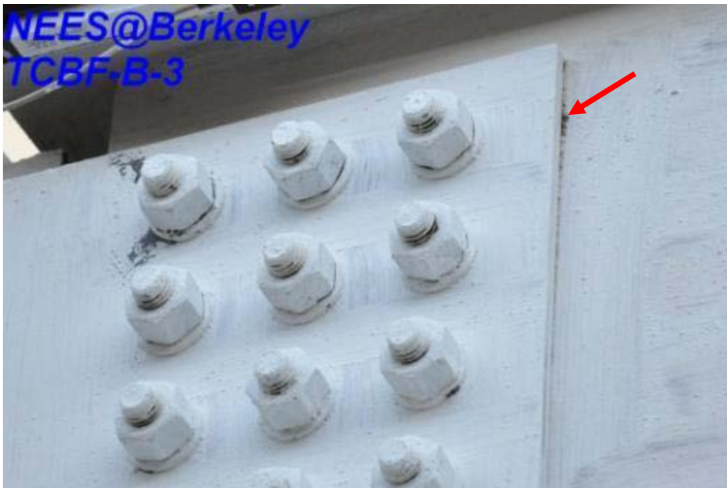
Figure 4.320 Evidence of slippage between splice plate and the one-piece gusset plate
