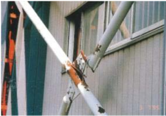
(a) Connection failure in a single-story X braced frame using round HSS braces
