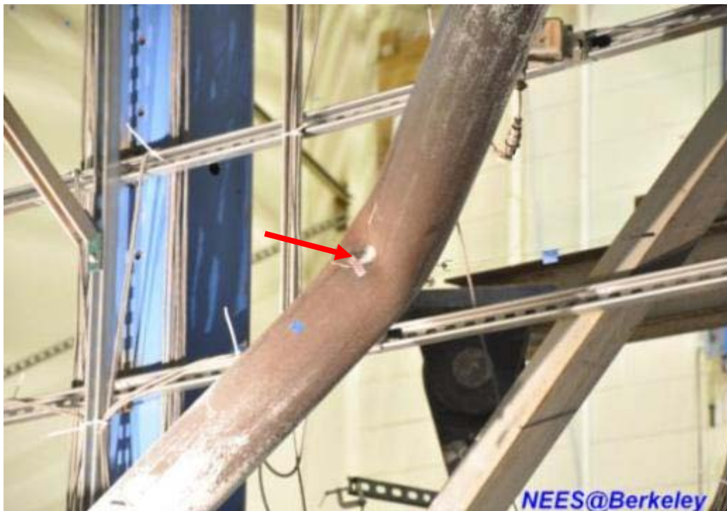
Figure 4.214 Additional local buckling of west side round HSS brace in the first story (Specimen TCBF-B-2)
