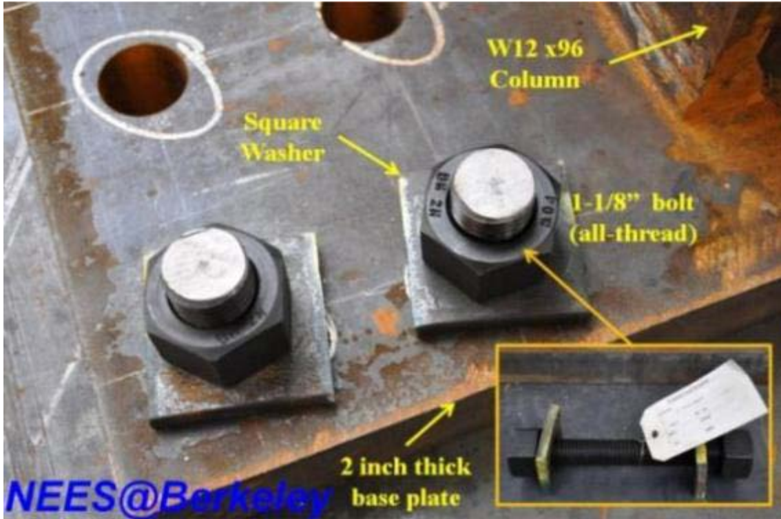
Figure 3.35 The 1-1/8 inch diameter all-thread anchor bolt
