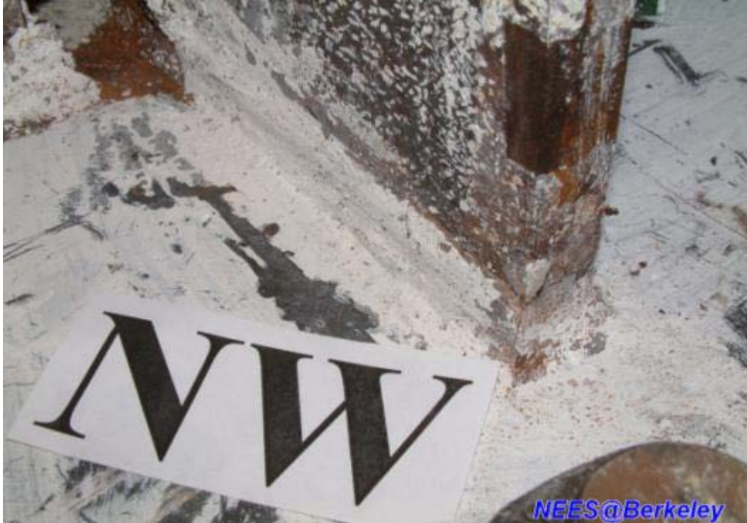
Figure 3.48(a) Crack in the CJP weld at west column base (north-west corner)
