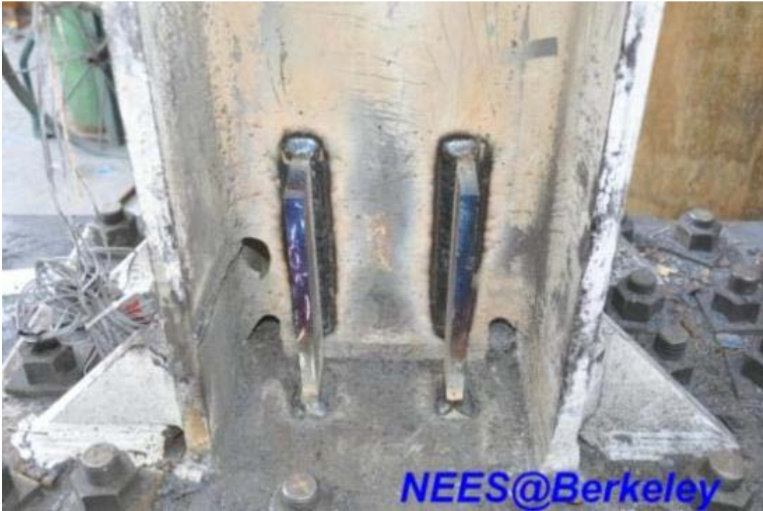
Figure 3.63 Two 0.55-in. thick vertical stiffener plates welded to the north face of column web with fillet welds at east side W12 × 96 column base
