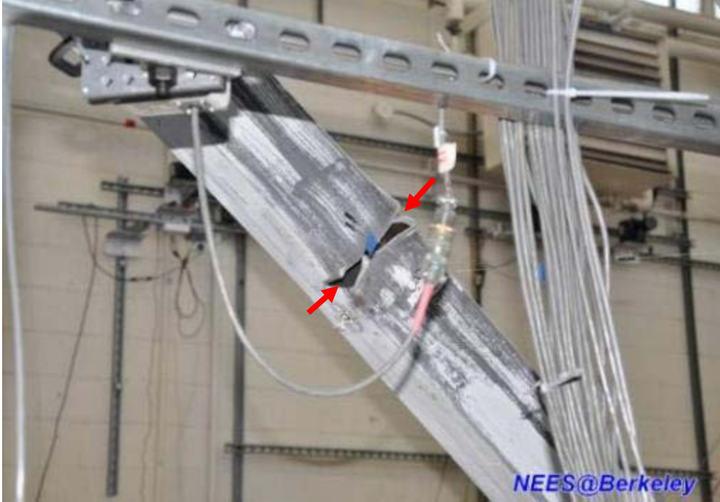
Figure 4.96 The cracks propagate in the square HSS brace at first story western side of TCBF-B-1 specimen
