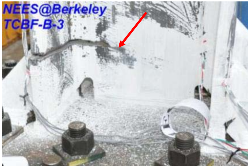
Figure 4.327 Crack tip in the web of east column near the column base
