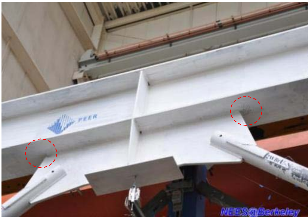
Figure 4.196 Whitewash flaking at the corner of gusset plate-to-roof beam connection (Specimen TCBF-B-2)
