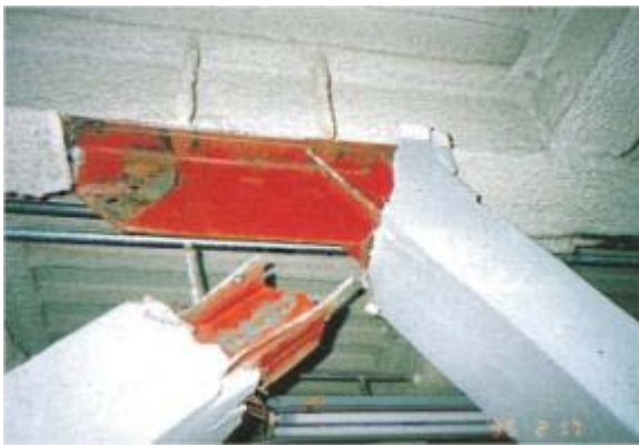
(a) Bolt failures in a double channel brace-to-gusset plate connection
