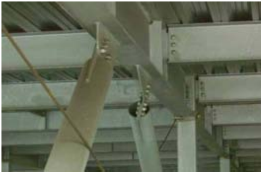
(c) Gusset plate buckling in a two-story parking structure
