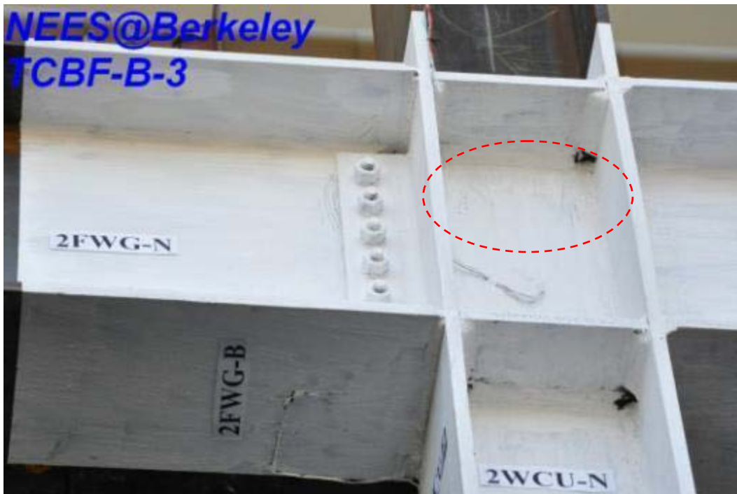
Figure 4.312 Whitewash flaking at the roof beam-to-column connection (west side)
