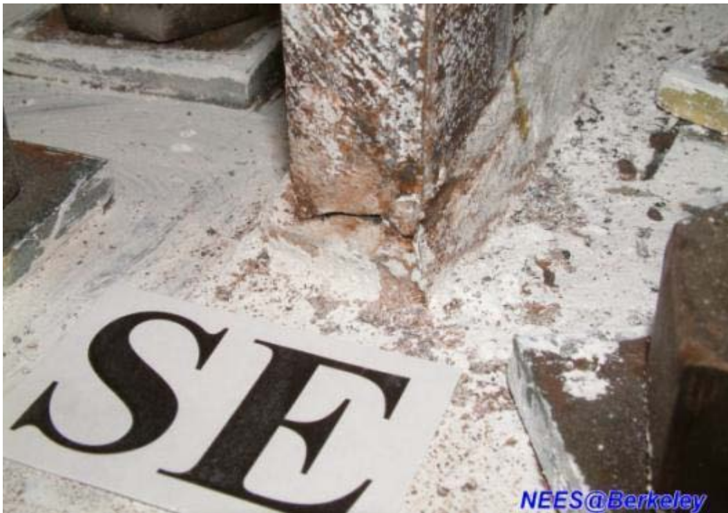
Figure 3.48(b) Crack in the CJP weld at east column base (south-east corner)
