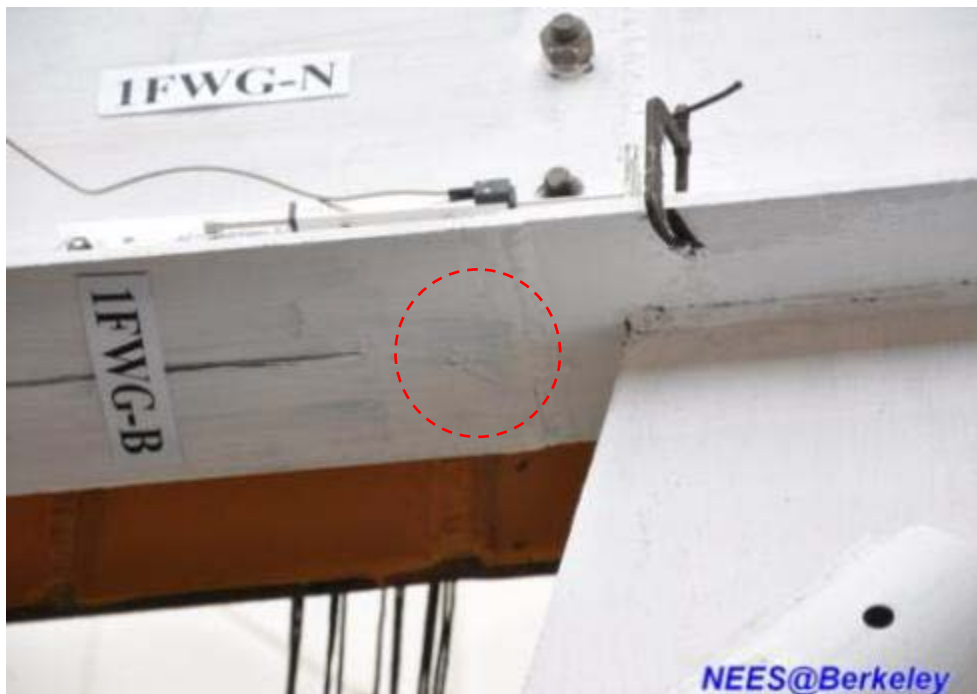
Figure 4.190 Flaking of whitewash near the CJP welds in the bottom flange of lower beam (Specimen TCBF-B-2)
