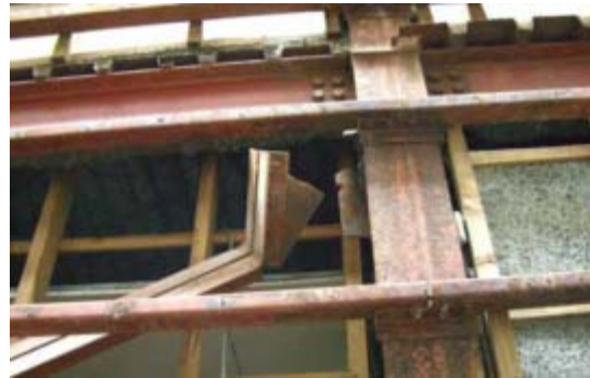
(d) Gusset plate net section failure in a low-rise industrial building
