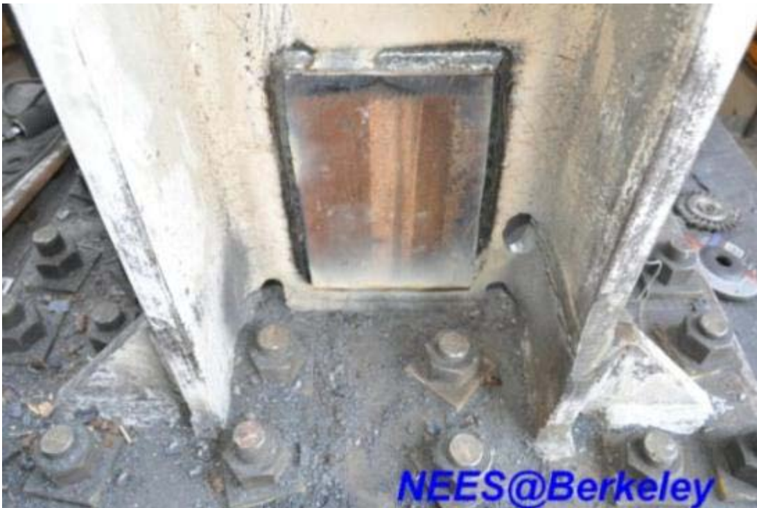
Figure 3.62 A 0.55-in. thick cover plate welded to the south face of column web with fillet welds at east side W12 × 96 column base
