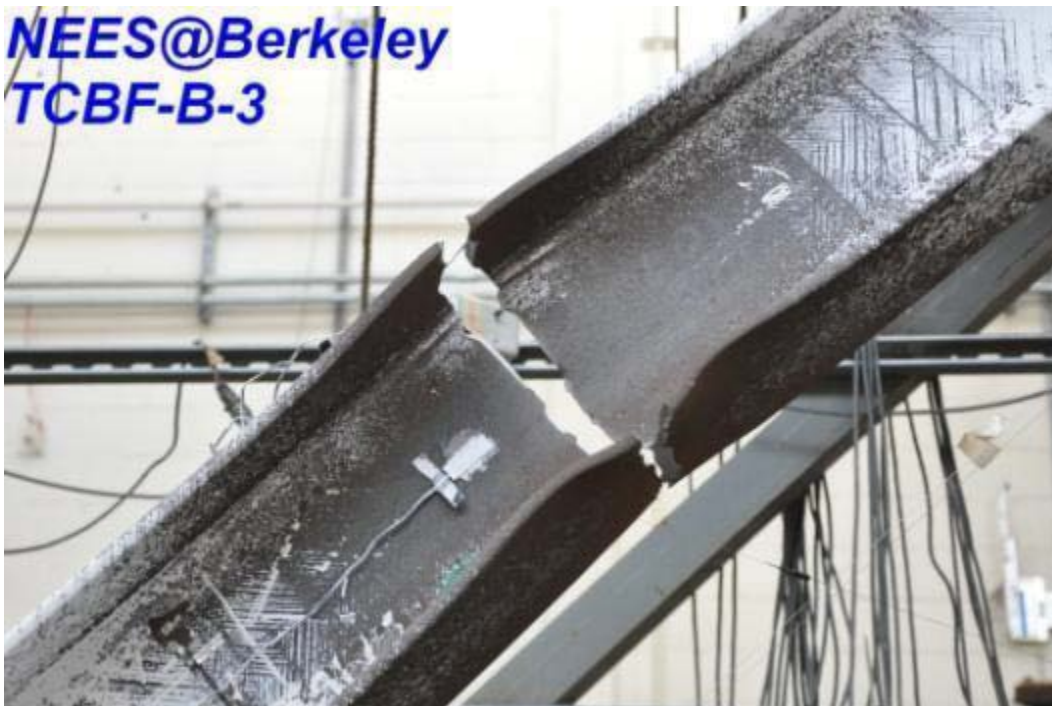
Figure 4.326 West wide flange brace completely fractured near the middle of the brace (view from north side)
