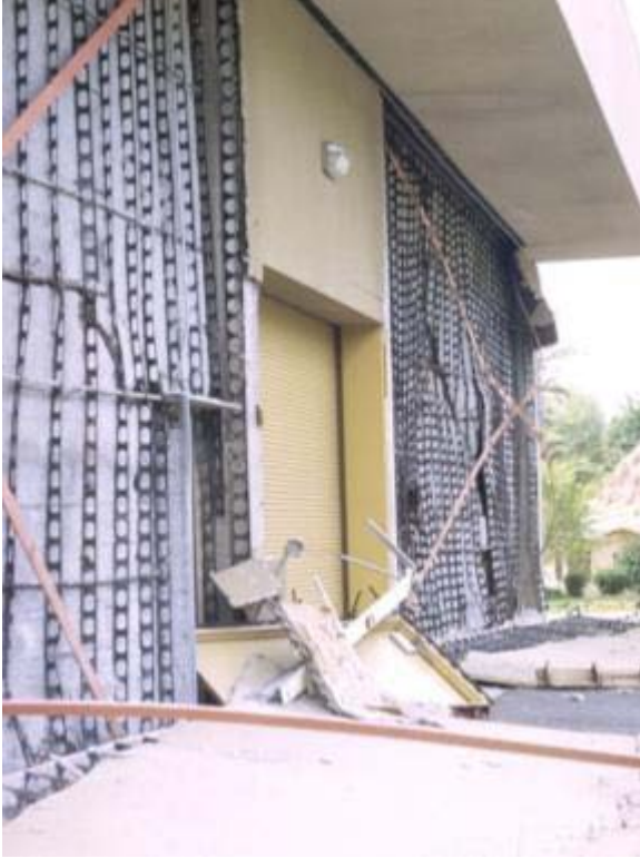
(a) Out-of-plane buckling of steel flat-bars (source: NISEE e-Library by Steinbrugge, Karl V.)
