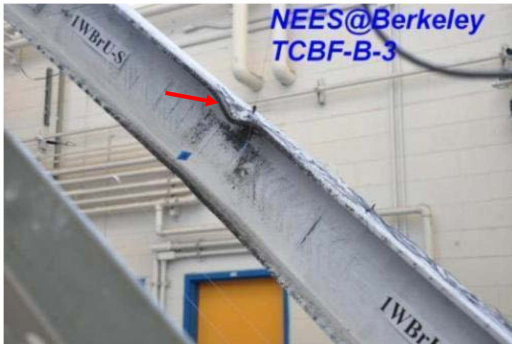
Figure 4.318 The closed view of flange local buckling at the west-side wide flange brace in the first story
