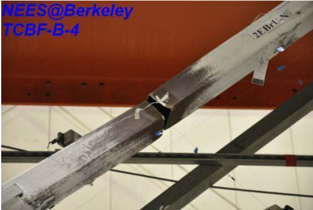
Figure 4.424 Completely fracture of the second story eastern side brace
