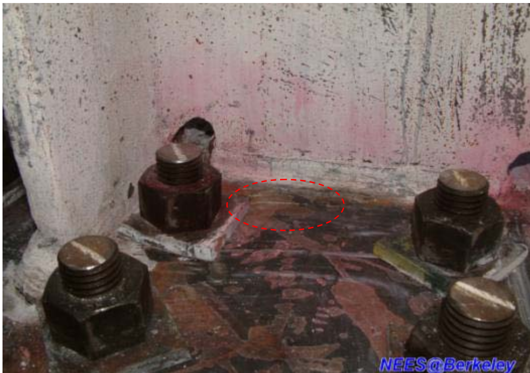
Figure 4.202 Crack near the web CJP welds at west side column base (Specimen TCBF-B-2)
