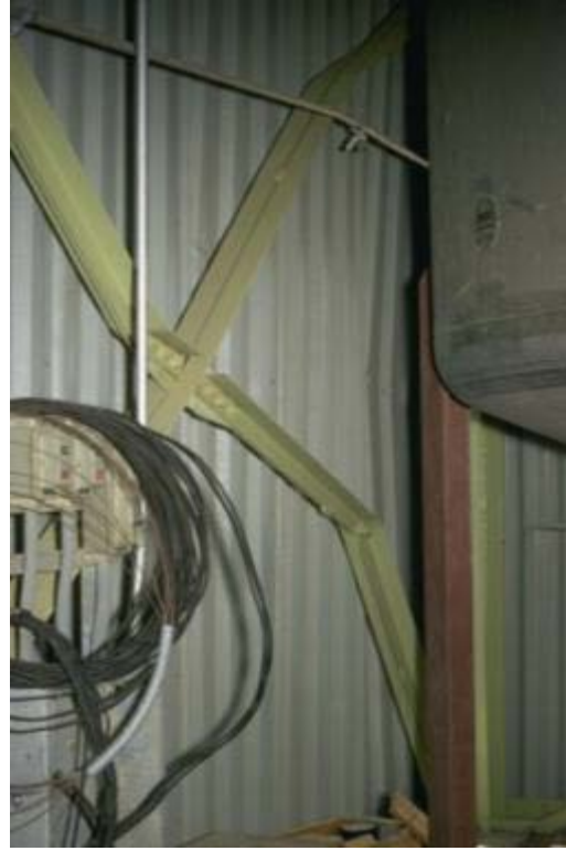
(b) In-plane buckling of double-angle braces (source: NISEE e-Library by Steinbrugge, Karl V.)
