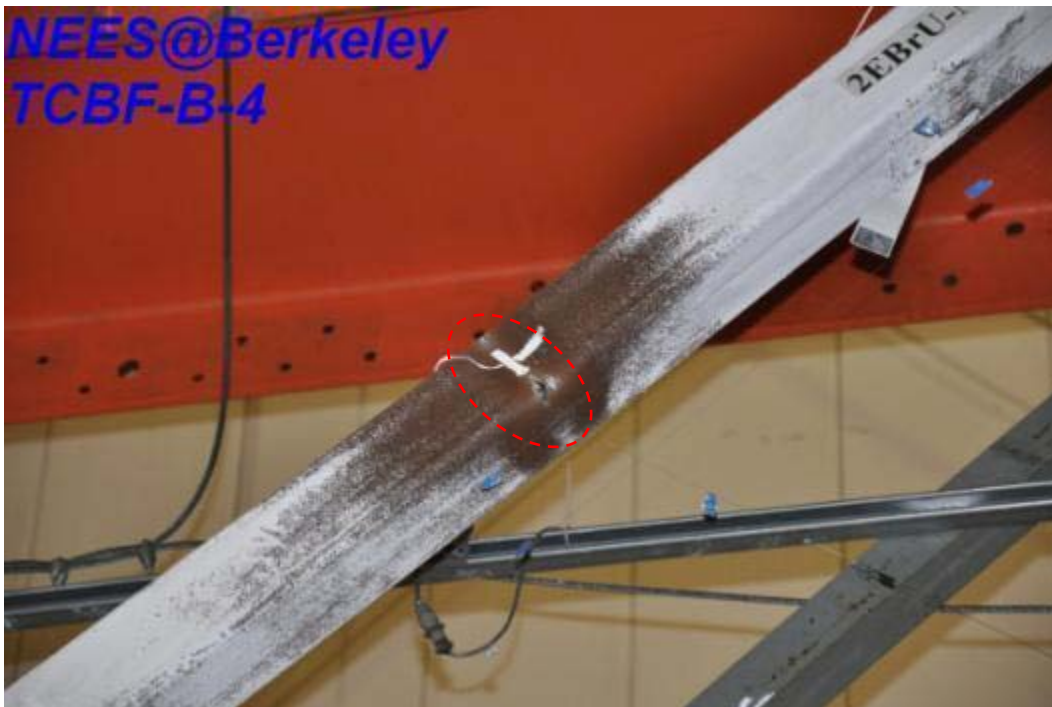
Figure 4.423 Cracks opening in the second story eastern brace
