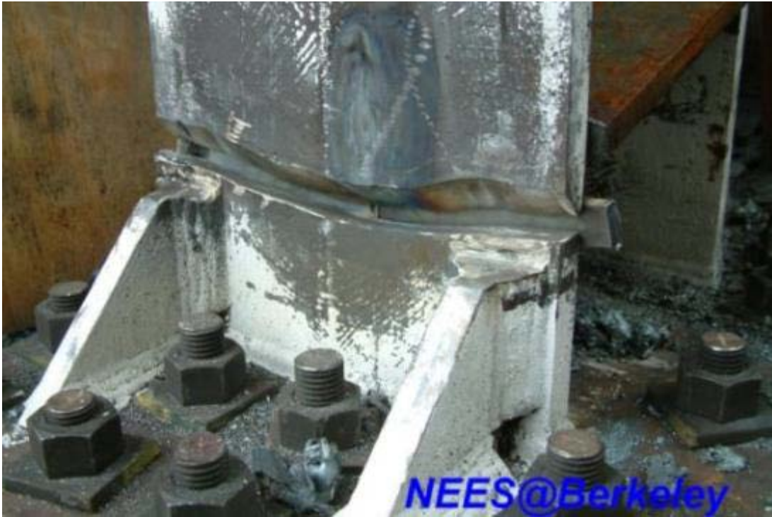
Figure 3.61 Grove prepared in the east side column flange near column base
