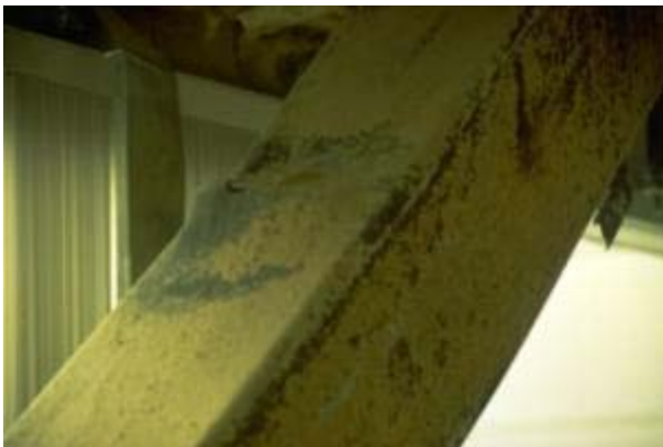
(a) Local buckling of square HSS brace section wall (source: NISEE e-Library)
