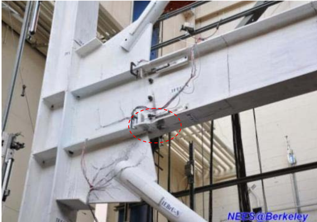
Figure 4.197 Local buckling of lower beam bottom flange at east side (Specimen TCBF-B-2)
