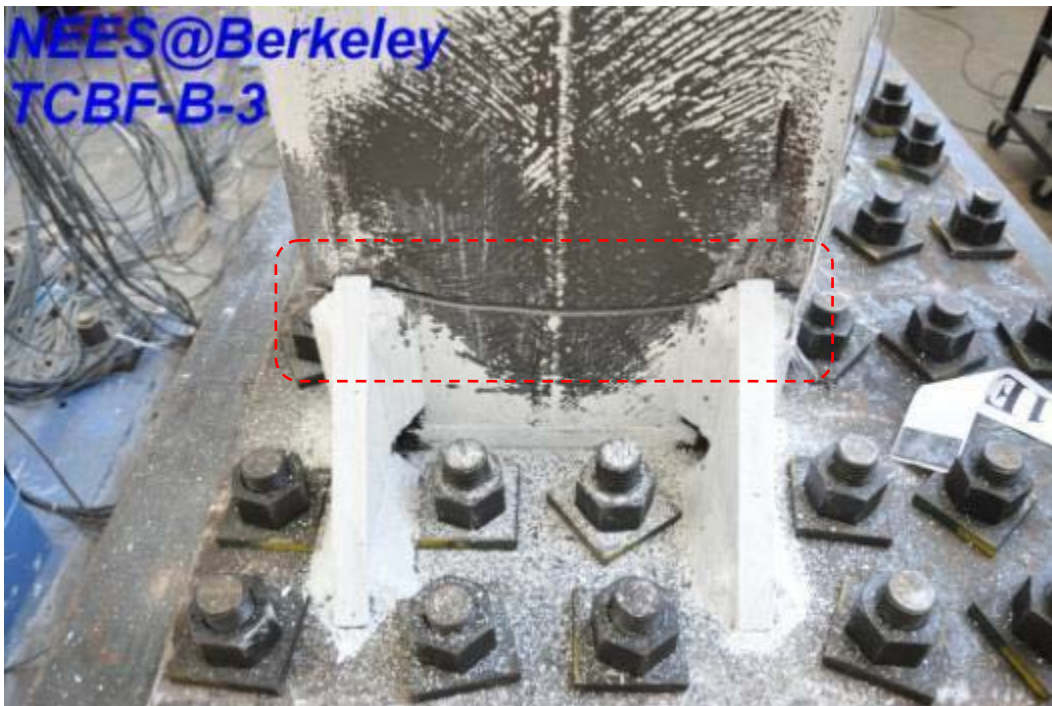
Figure 4.322 East column flange fractured near the base plate stiffeners (view from east side)
