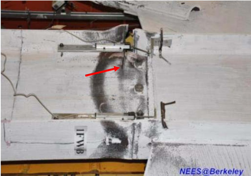
Figure 4.220 Crack in the lower beam web at west side near top flange (Specimen TCBF-B-2)
