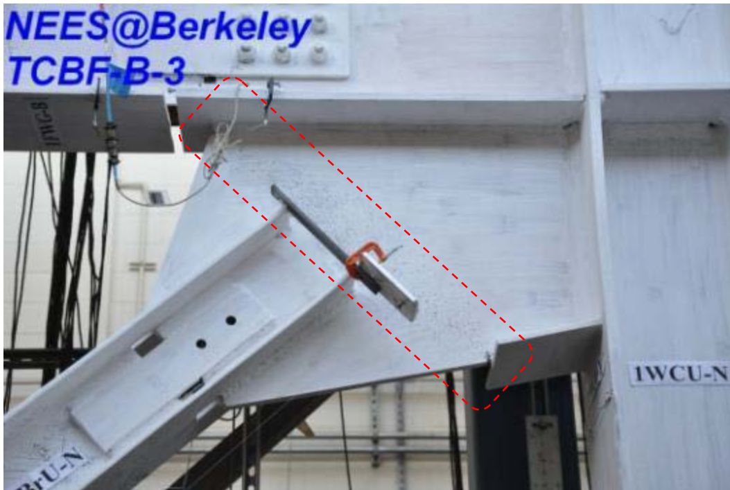
Figure 4.315 Flaking of whitewash developed at the 2t gap region in the gusset plate
