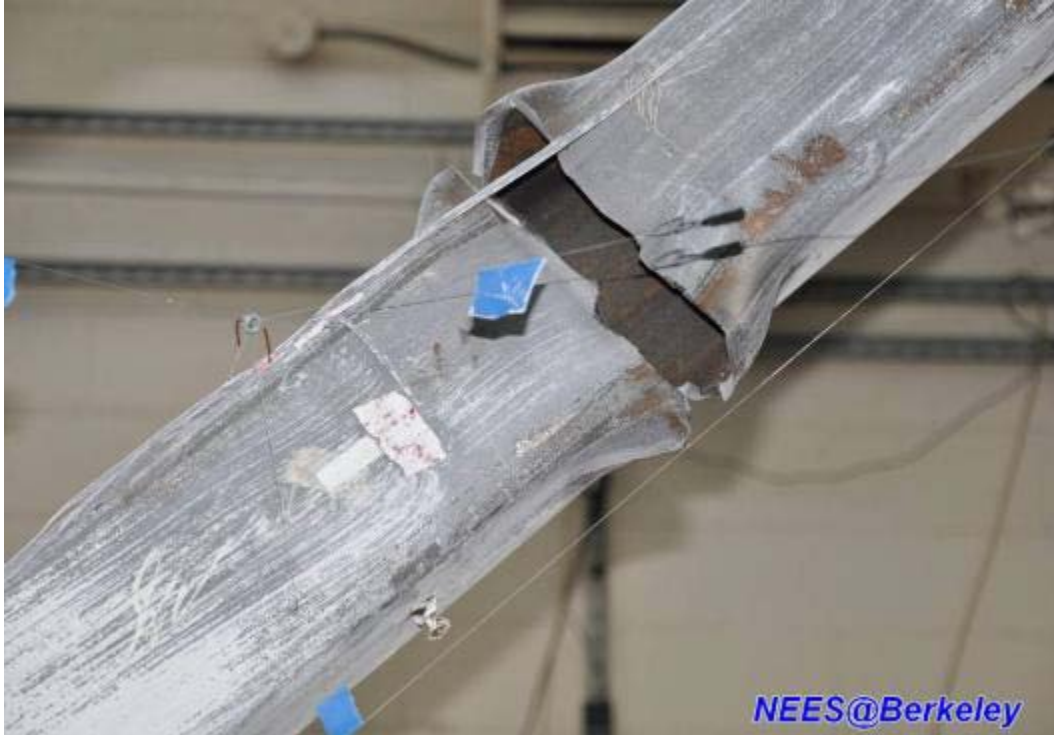
Figure 4.100 Complete fracture of the square HSS brace at first story eastern side of TCBF-B-1 specimen
