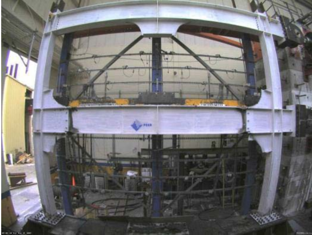
Figure 3.43 Damaged specimen after cutting off the square HSS braces
