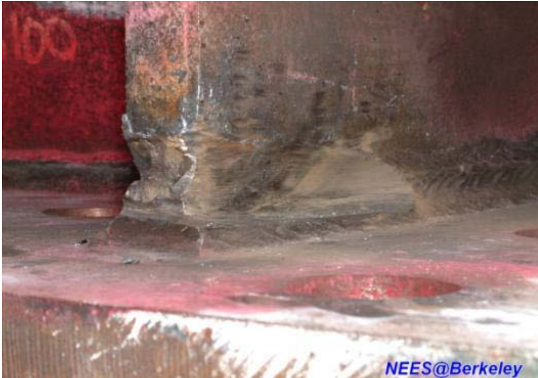
Figure 3.51 The east column base (south-east corner) after gouging the cracked welds
