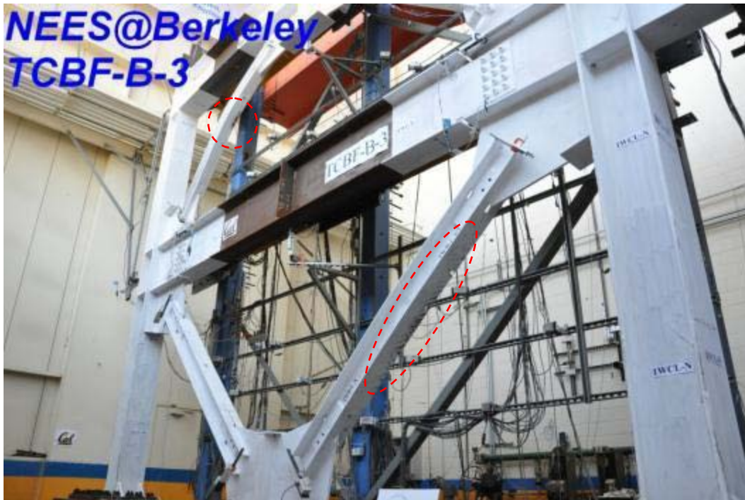
Figure 4.311 Whitewash flaking on the global buckled braces (west brace at the first story and east brace at the second story)
