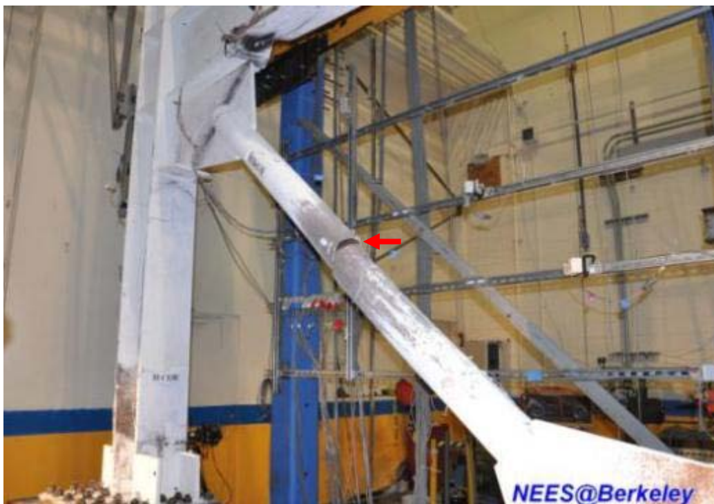
Figure 4.224 Complete fracture of the east side brace in the first story (Specimen TCBF-B-2)
