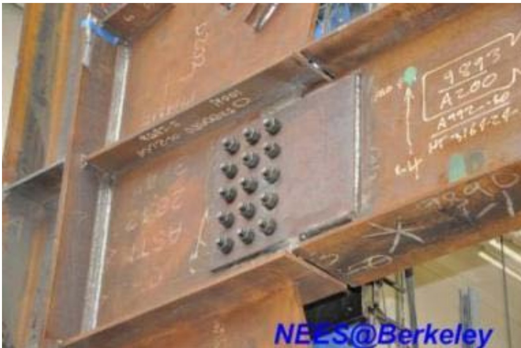
Figure 4.227 The lower beam to one-piece gusset plate pin connection detail of TCBF-B-3 specimen (eastern side of the W24 x 68 beam)
