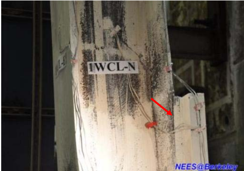
Figure 4.217 Additional tearing of fillet welds between cover plate and column flange (Specimen TCBF-B-2)
