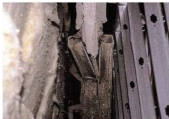
(b) Weld failures at brace-to-gusset plate connection (source: EERI, 1997)
