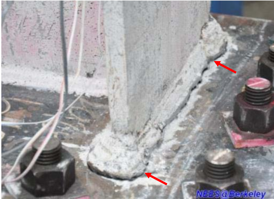
Figure 4.103 Fracture of the column base flange CJP welds at west side of TCBF-B-2 specimen
