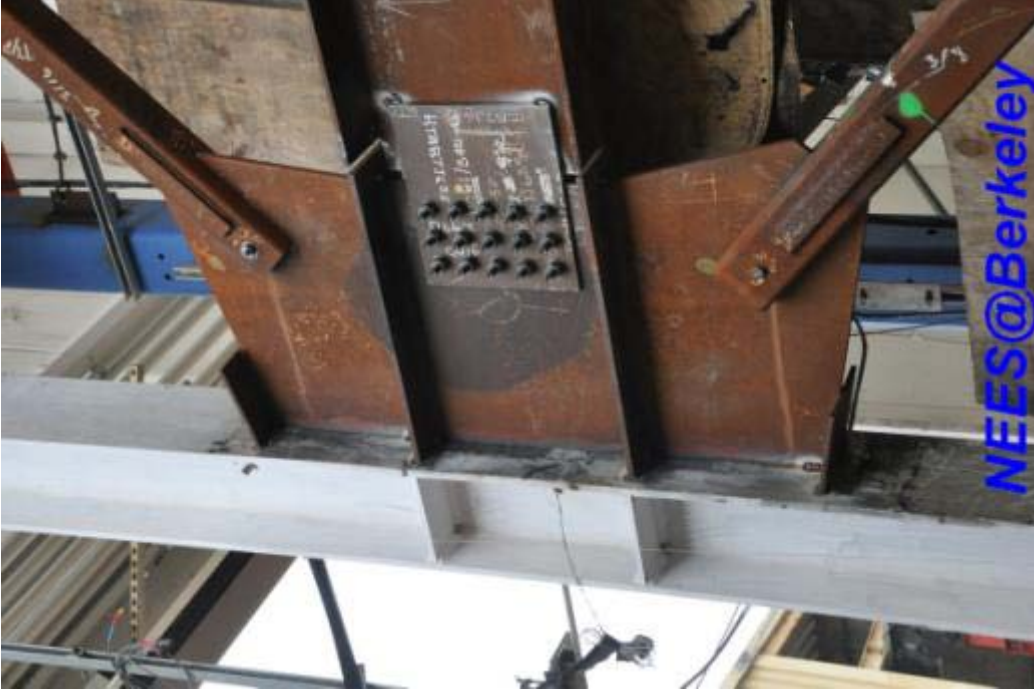
Figure 3.60 Connection detail of the lower beam to one-piece gusset plates of TCBF-B-4 specimen
