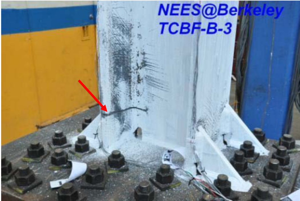
Figure 4.321 East column flange fractured near the base plate stiffeners (view from north-west side)
