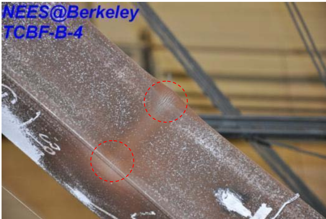
Figure 4.419 Cracks in the first story eastern side brace
