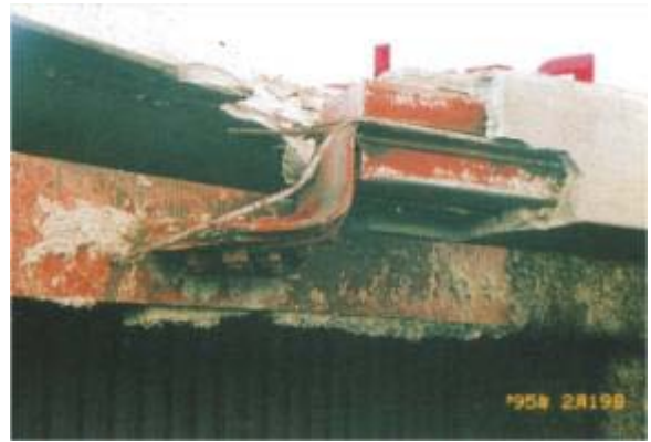
(b) Buckling of gusset plate
