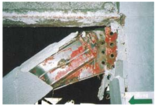
(b) Bolt failures in a gusset plate-to-column connection
