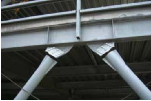
(a) Brace connection fractures in a two-story parking structure
